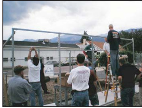
Apprentices with the Joint Apprenticeship Training Committee learning to install solar panels.
