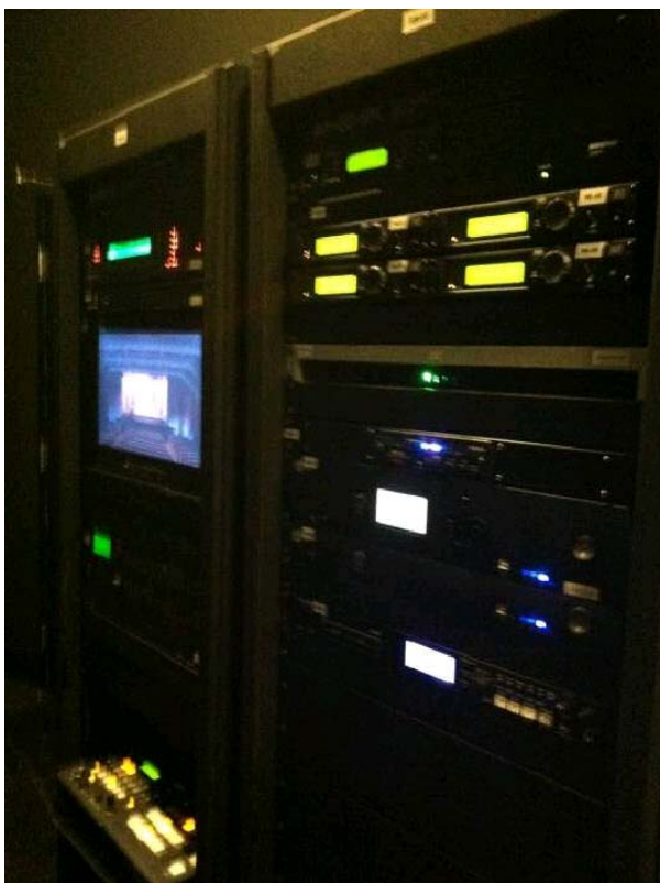
Figure 2. A/V tele-conference equipment for the NCWCP auditorium
