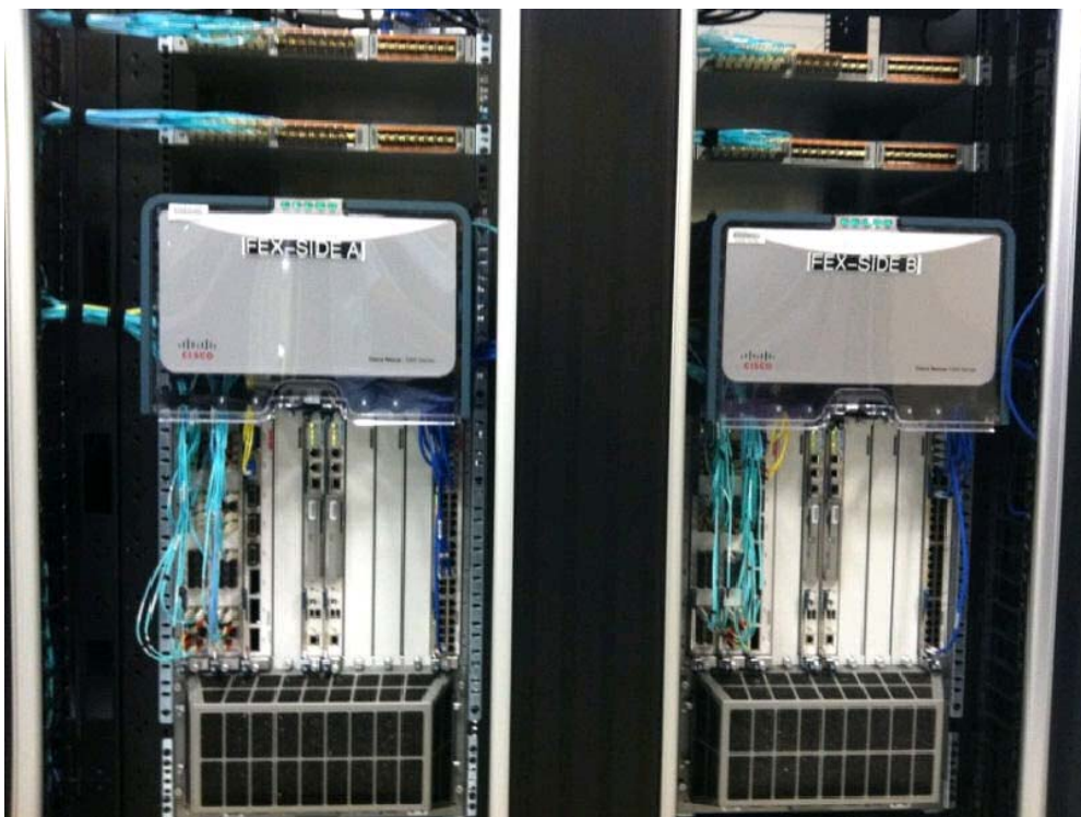
Figure 1. Redundant core routers connecting the NCWCP and its wide area network
