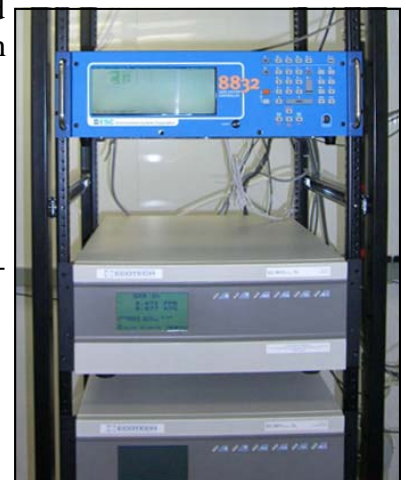
Air Monitoring Equipment
