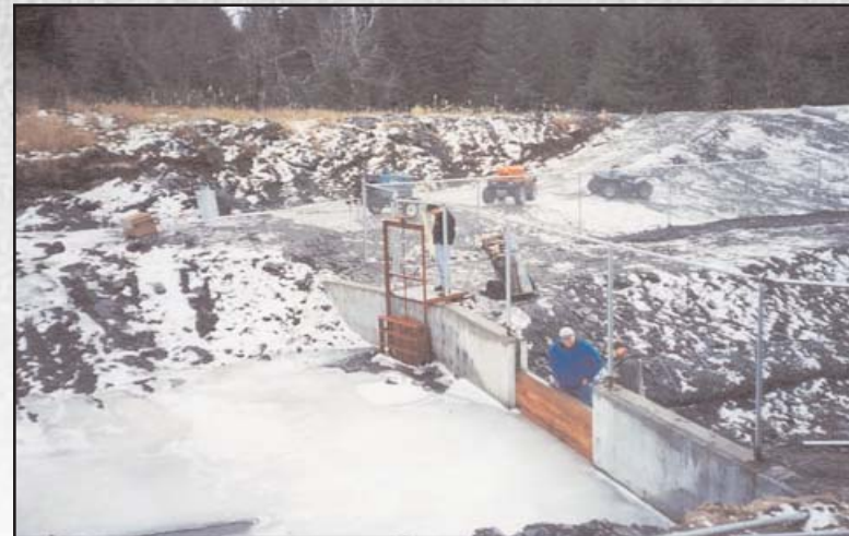
Figure 41: Port Lions surface water impoundment, Alaska.
