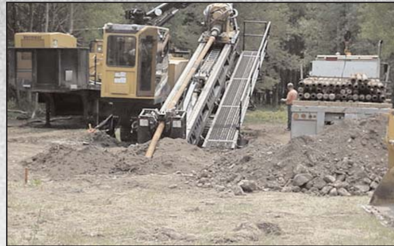
Figure 21: Drill rig boring the first pass with the 8 inch drill bit. Passes with a 24 and 26 inch drill bit will be required to install the 22 inch water main.
