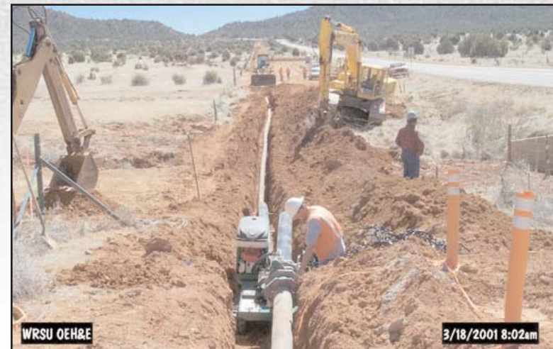
Figure 14: Over 12 miles of water transmission line was installed from Canyon Day to Cedar Creek.
