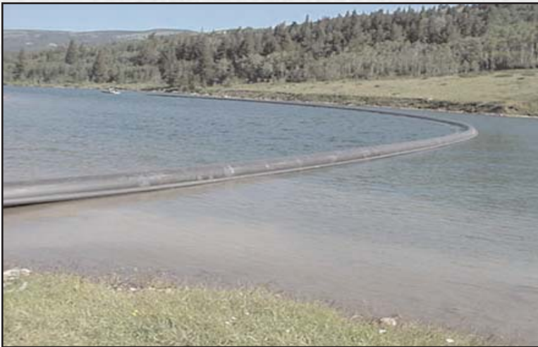
Figure 19: 22 inch HDPE pipe and 4 inch air line floating on the lake waiting to be pulled through the bore hole in the deep spot of the lake.
