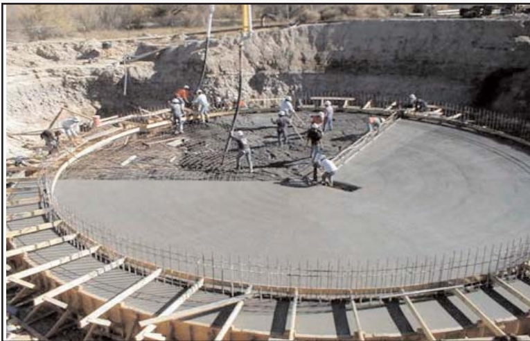
Figure 40: Concrete pour for a clarifier base on the Shiprock wastewater treatment plant.
