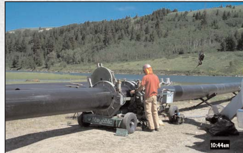
Figure 20: 22 inch HDPE pipe fused together for installation at the bottom of the lake.
