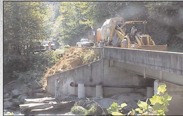
Figure 28: Straight Fork Bridge ductile iron sewer main.
