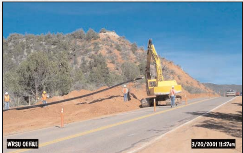
Figure 15: Transmission line installed in the White Mountains.
