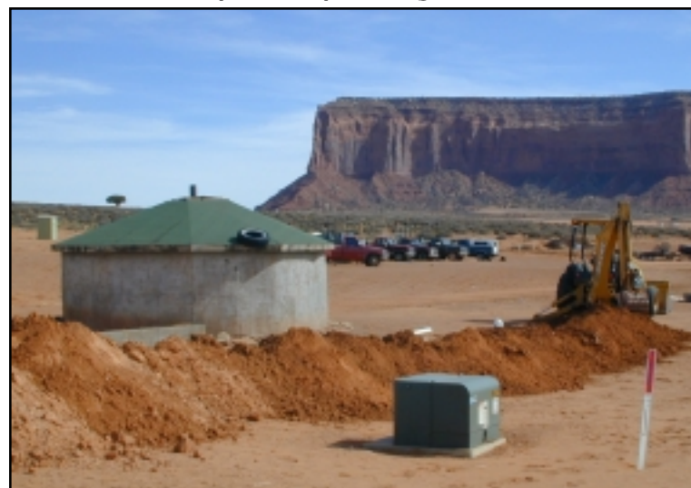
Figure 25: Bathroom addition and waterline construction at a hogan in Monument Valley, AZ.
