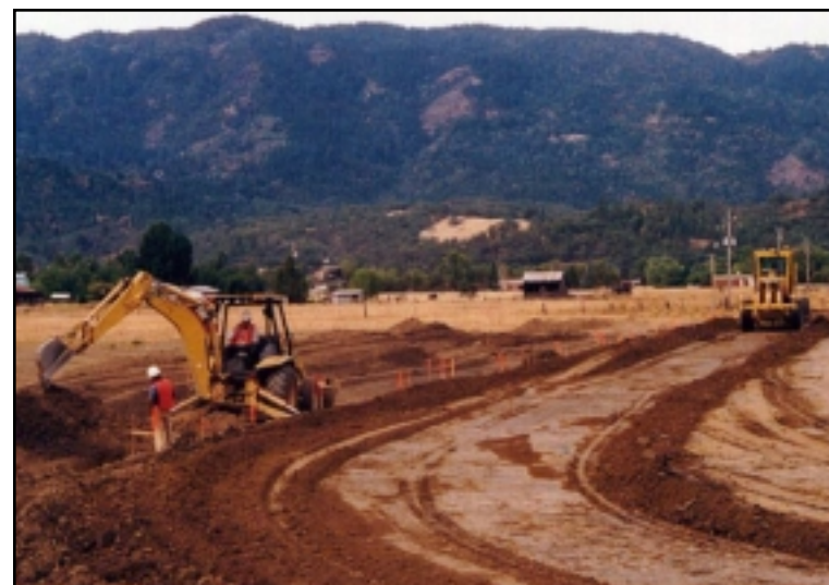
Figure 21: Construction of the south dike of the AIWPS outer treatment pond cell
