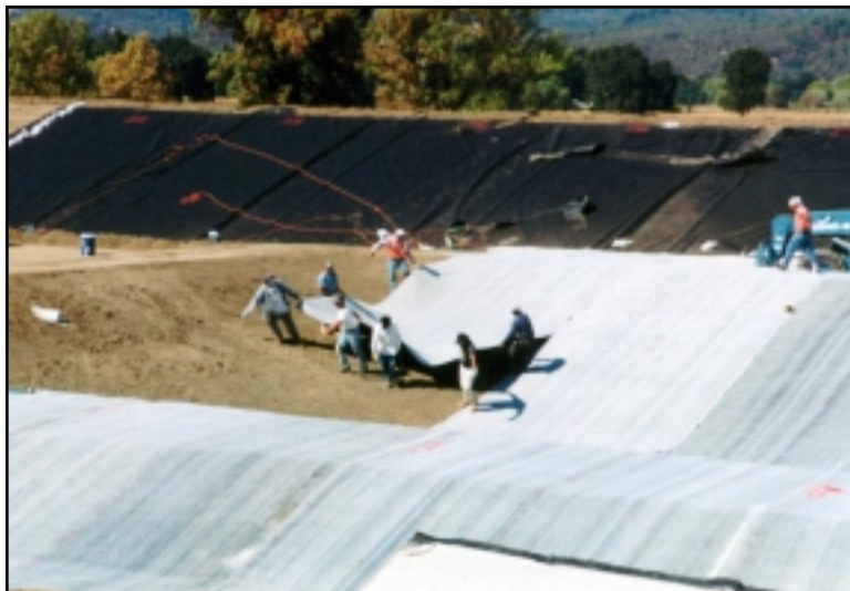
Figure 22: Installation of the Reinforced Geosynthetic Clay Liner(GCL) in the AIWPS Fermentation Cell Pit.
