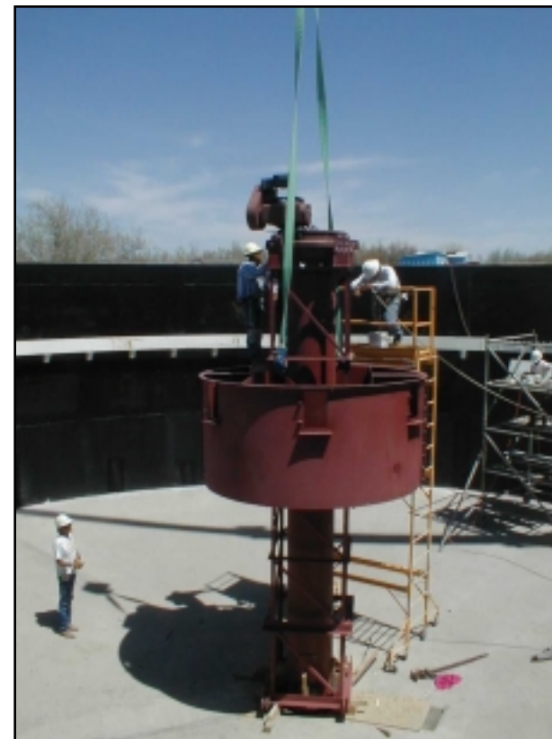
Figure 29: Clarifier mechanism drive unit on the center column.
