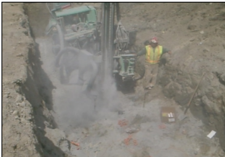
Figure 36: Drilling for rock removal to facilitate installation of water main, Bois Forte Reservation.
