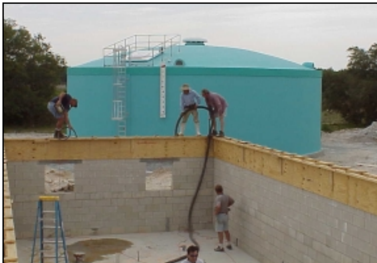
Figure 39: Construction of a pump station and ground level tank, Seminole Tribe, FL
