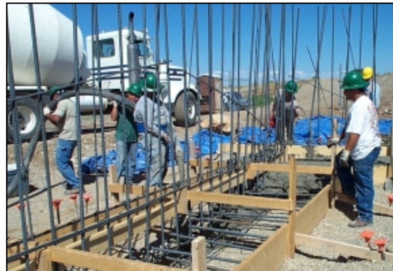
Figure 41: Tribal contractor preparing forms and reinforcement for solid waste transfer station at Taos Pueblo, NM
