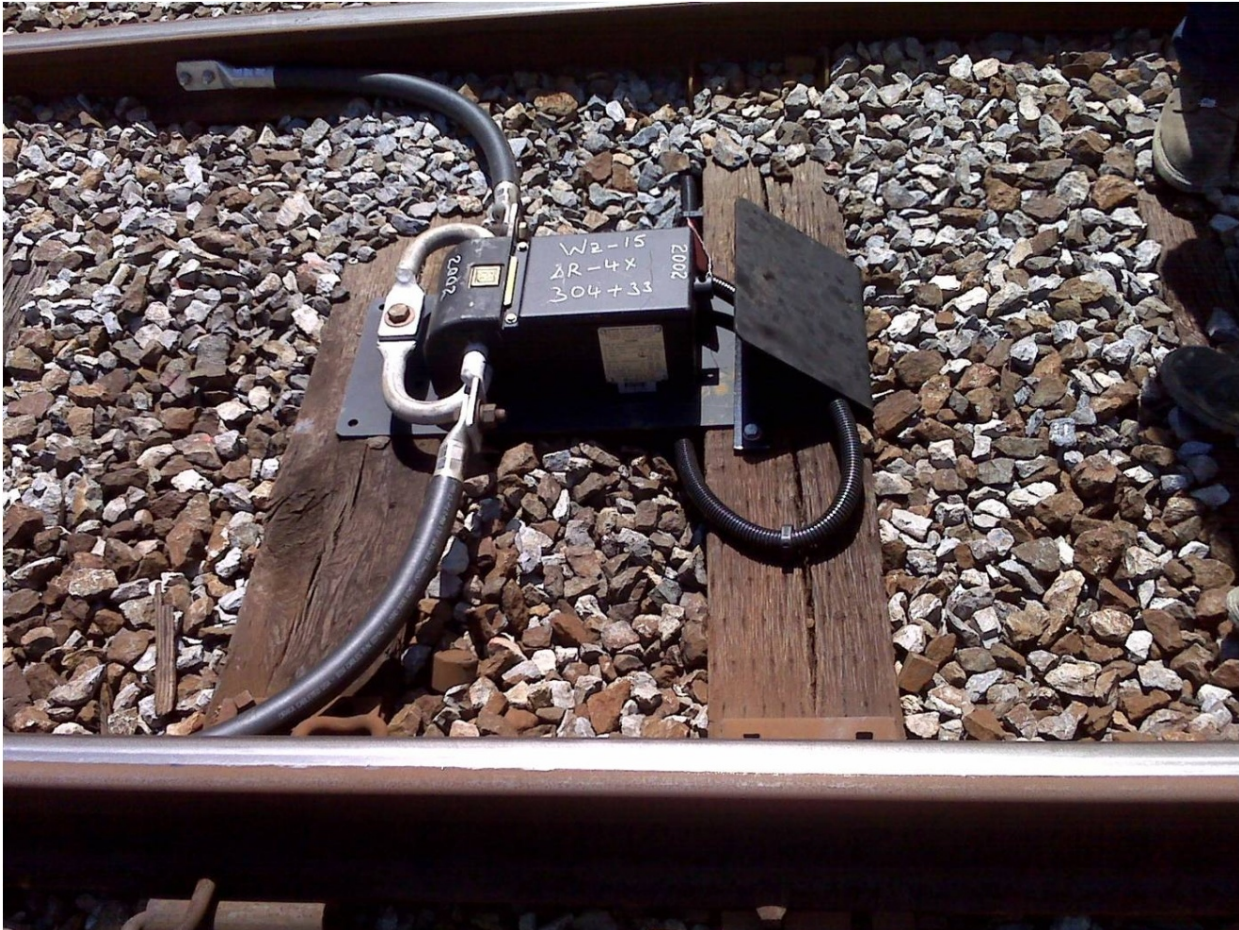
Figure 8. Impedance bond for track circuit B2-304.
