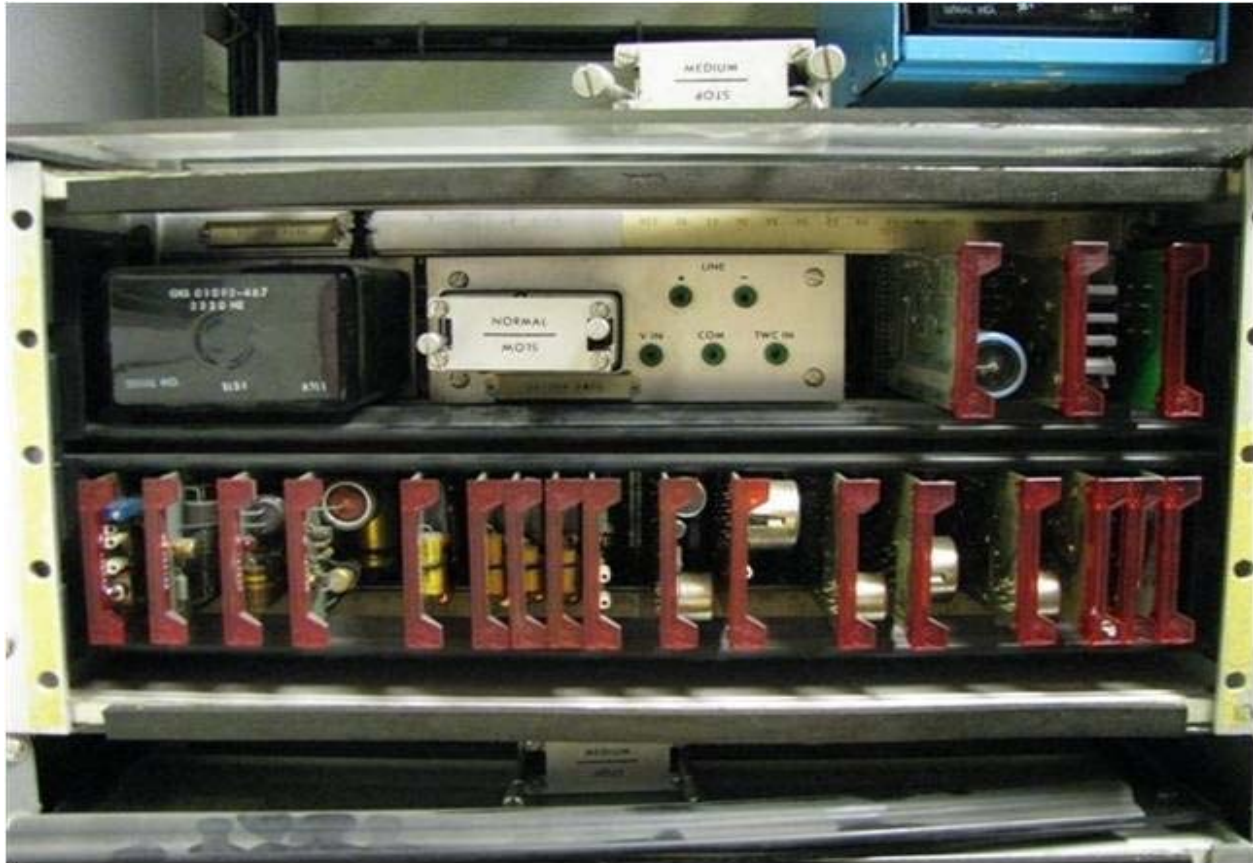
Figure 9. Typical track circuit module.
