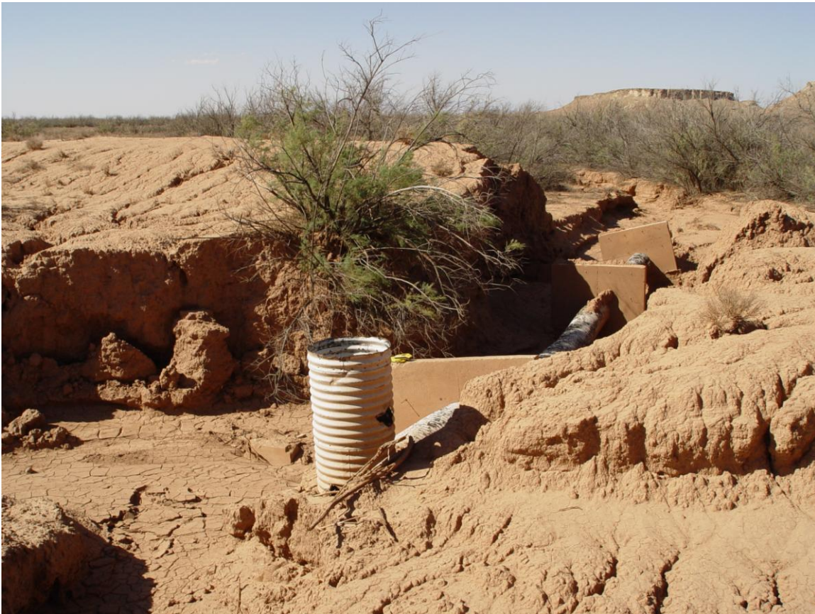
Figure 10 – Flat Top #1 overflow pipe exposed before repair
