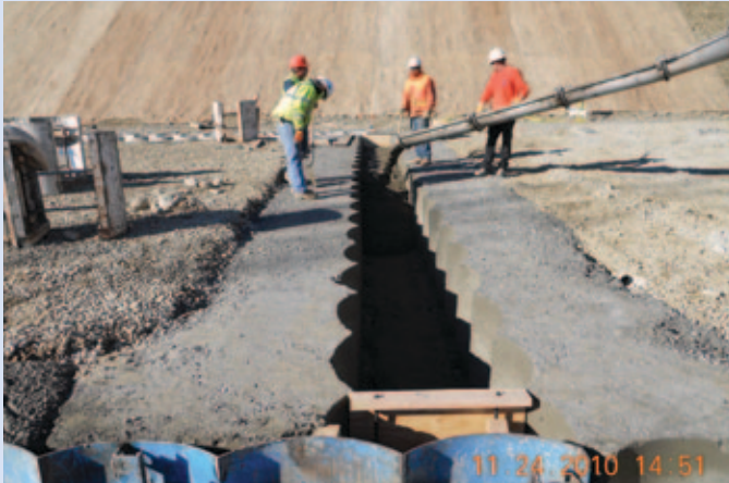
Initiation of modifications to Mormon Island Auxiliary Dam started in FY2010 with expected completion in 2014.
