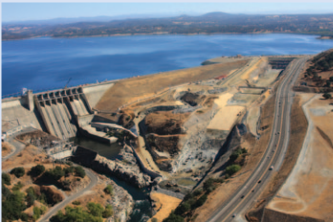
Phase II Spillway excavation nearing completion in FY 2010. The USACE will begin work on the JFP in FY 2011, with expected completion in 2015.
