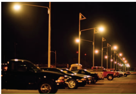
Photovoltaic-powered lights are installed in several parking lots at Fort Hood, Texas, in the largest lighting project of this kind in America. Photo from Solar Outdoor Lighting, NREL/PIX 07839
