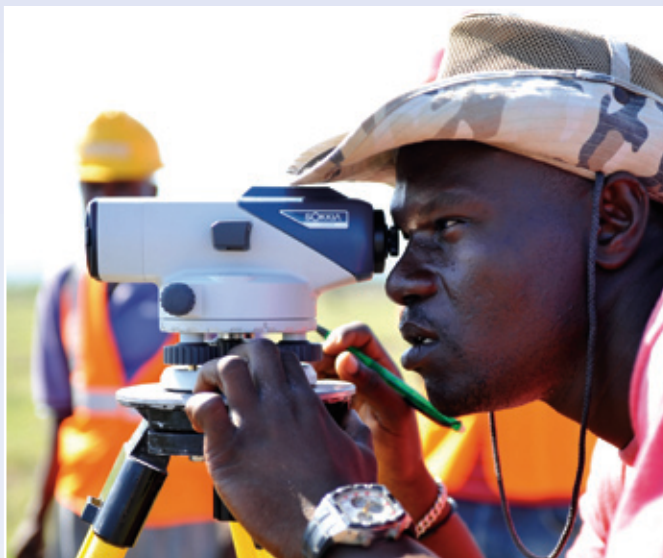
A worker surveys USAID-funded housing site near the Caracol Industrial Park in northern Haiti on November 10, 2011. USAID
