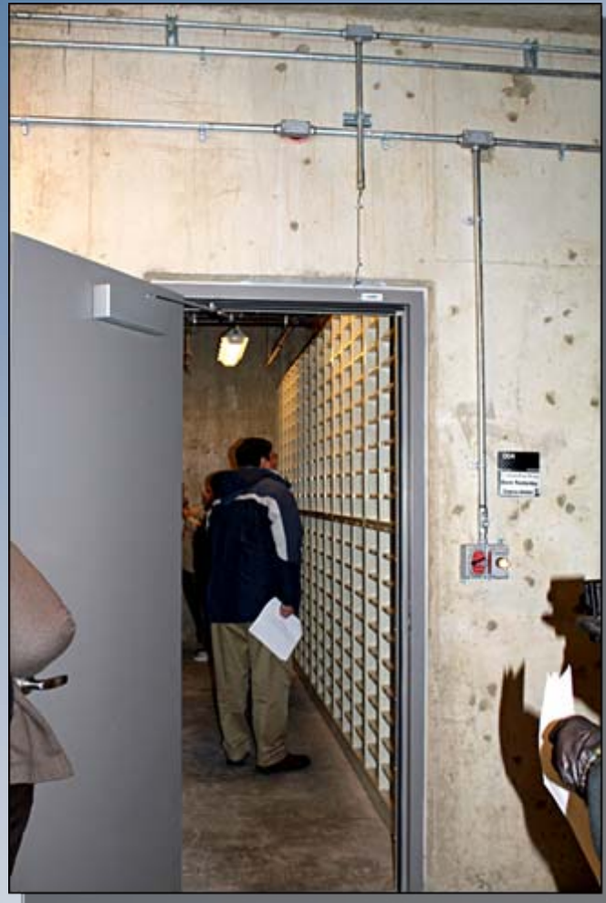
A federal librarian reviews the storage capability in one of the nitrate vaults.
