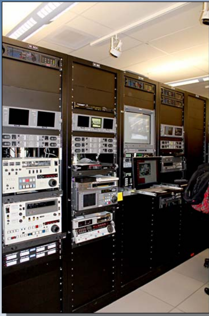
One of the third floor preservation systems.
