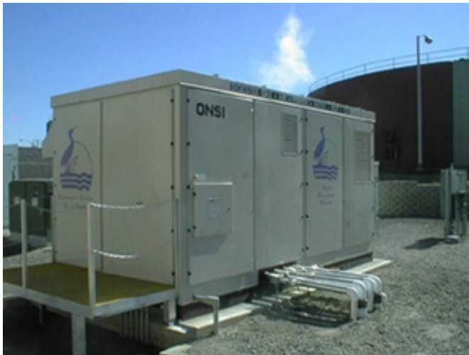
Figure 5-1. 200 kW ADG Fuel Cell in Portland, Oregon
