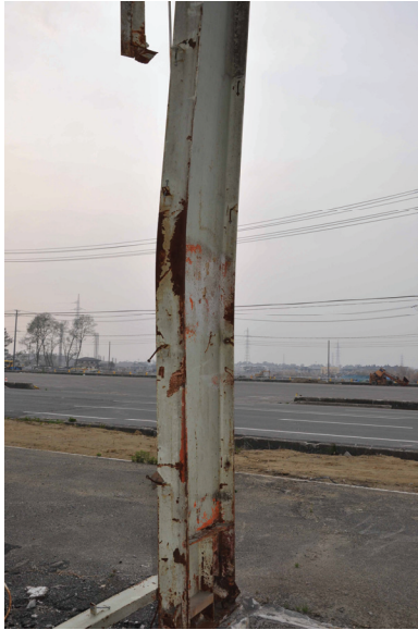
Figure A-12 Flexural buckling of a steel wide flange column (courtesy of D. Lignos).
