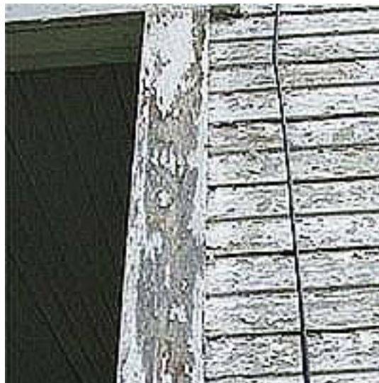
Paint Peeling on a House
