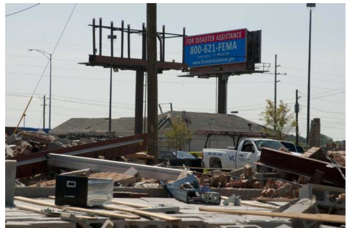
Tuscaloosa, Alabama, May 6, 2011 -- High above the catastrophic damage wrought by an F5 tornado, an operational electronic billboard flashes important assistance information to survivors.
