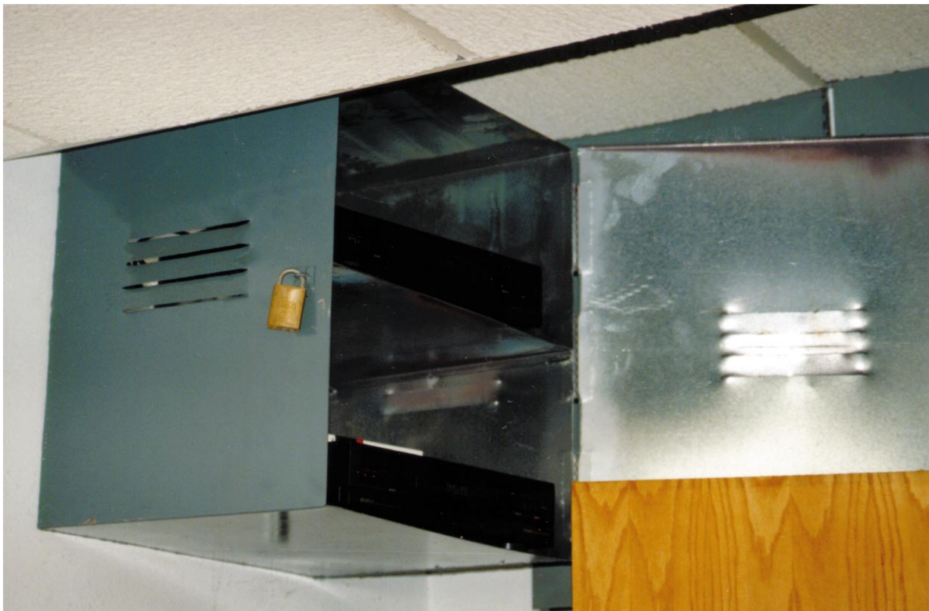
Exhibit 2.15. This video recording equipment is protected by a simple locked and vented cabinet that resides within a locked room.
