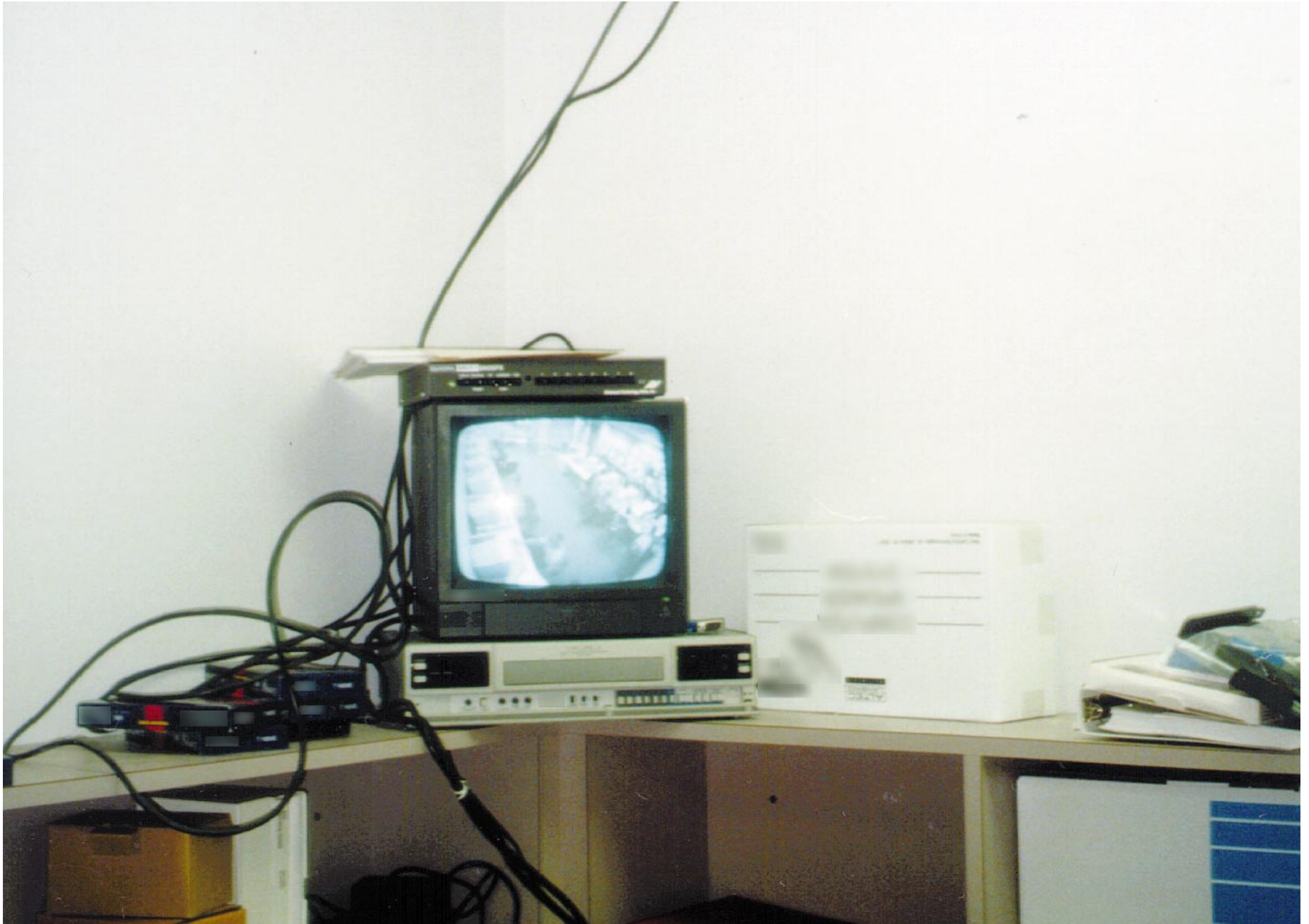
Exhibit 2.14. This is an example of a sloppy installation job—be careful how you word a contract for installation.
