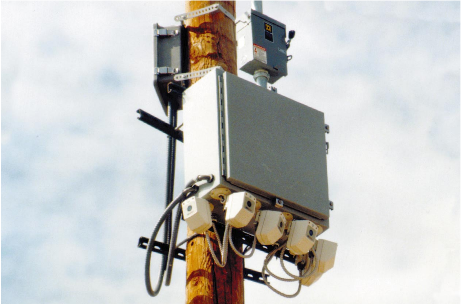
Exhibit 2.8. These bullet-resistant cameras on the light pole of a school parking lot were installed using wireless technology for data transmission. This configuration, which required line of sight between the transmitter and receiver, greatly reduced the expense and difficulty in running protected cabling back to the recording equipment. Note the protective shielding for the power cables that serve each camera.
