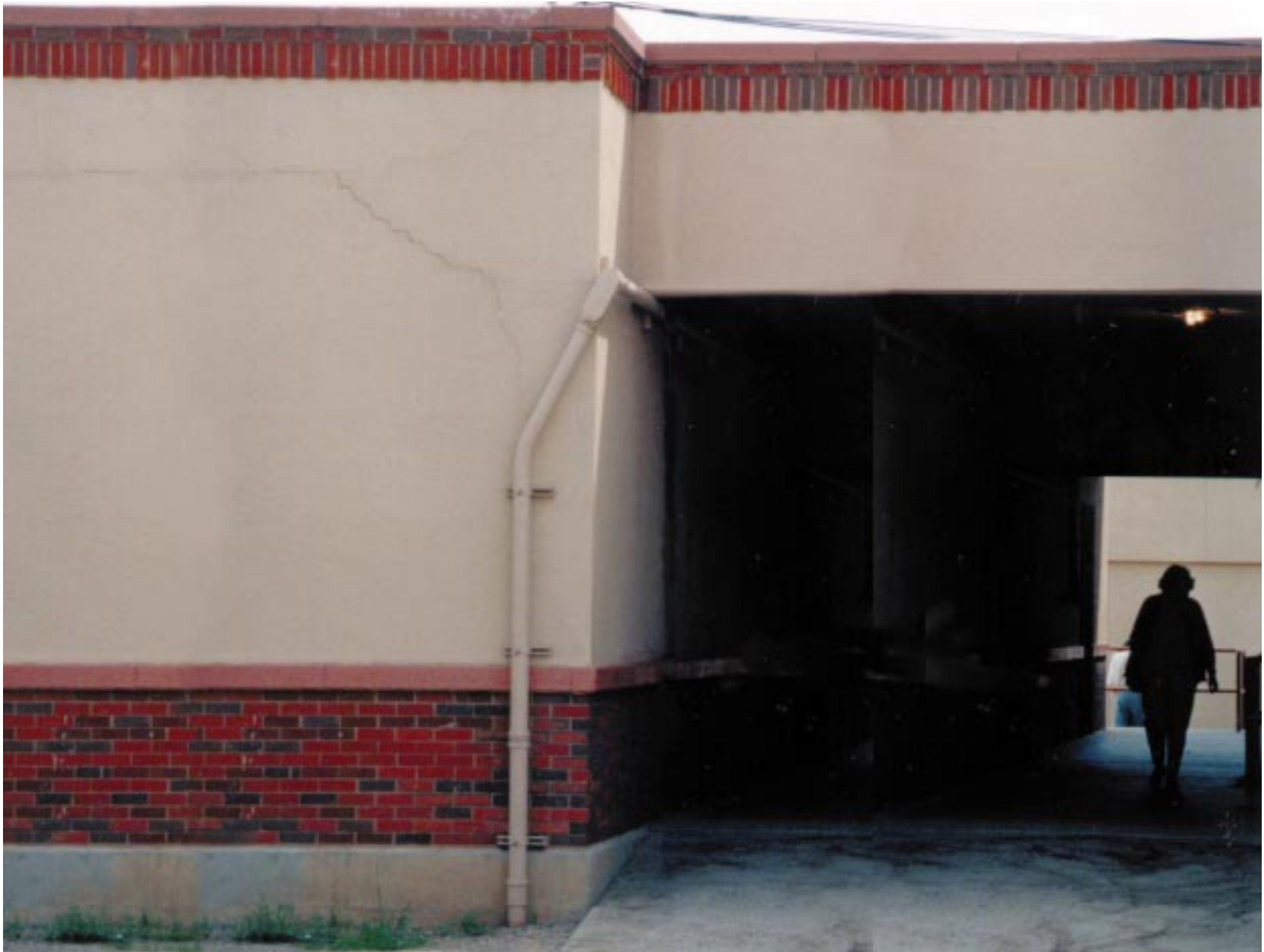
Exhibit 1.5. Be aware that exposed utility conduits or drain pipes can allow easy access to a school's roof, creating an opportunity for theft, as well as a liability concern.
