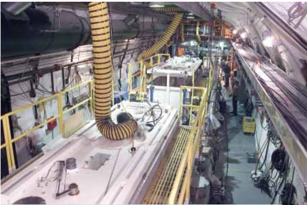
ASSURING STOCKPILE SAFETY: Cygnus is the machine that generates the power for the 2.5 MeV radiography pictures taken of the subcritical experiments.
