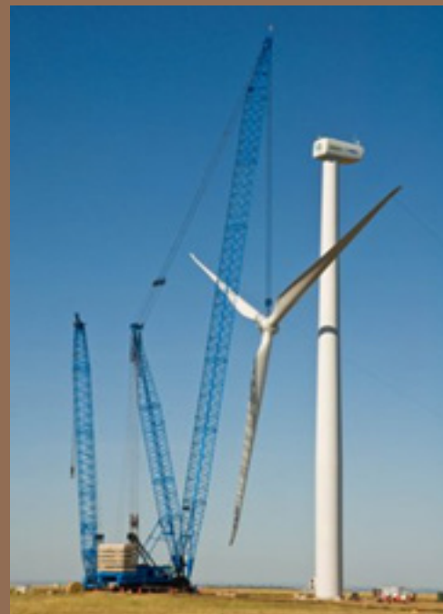
Installation of a 1.5 MW wind turbine at the National Wind Technology Center in Colorado. (source: National Renewable Energy Laboratory)
