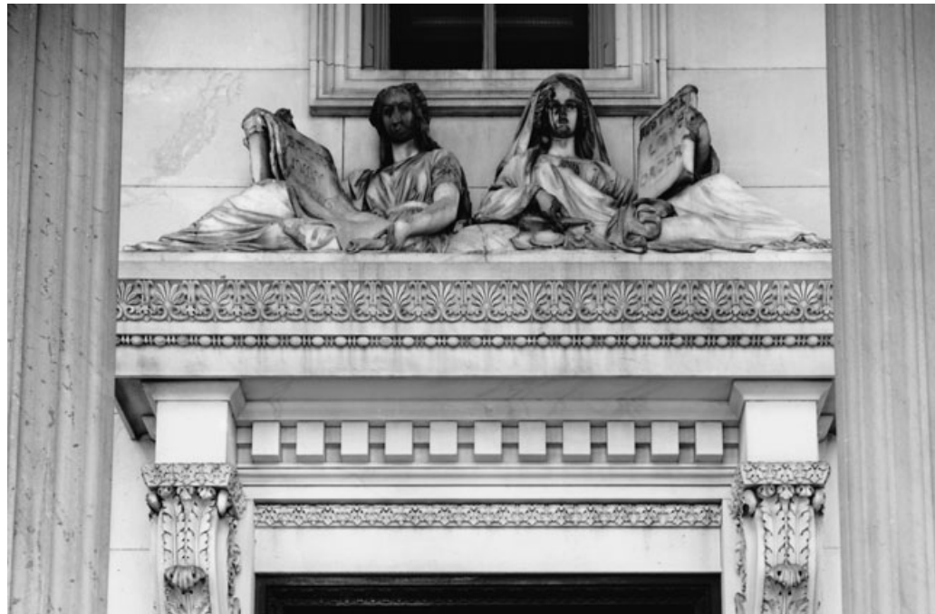
Justice and History with extensive deterioration evident, 1957. (Architect of the Capitol)
