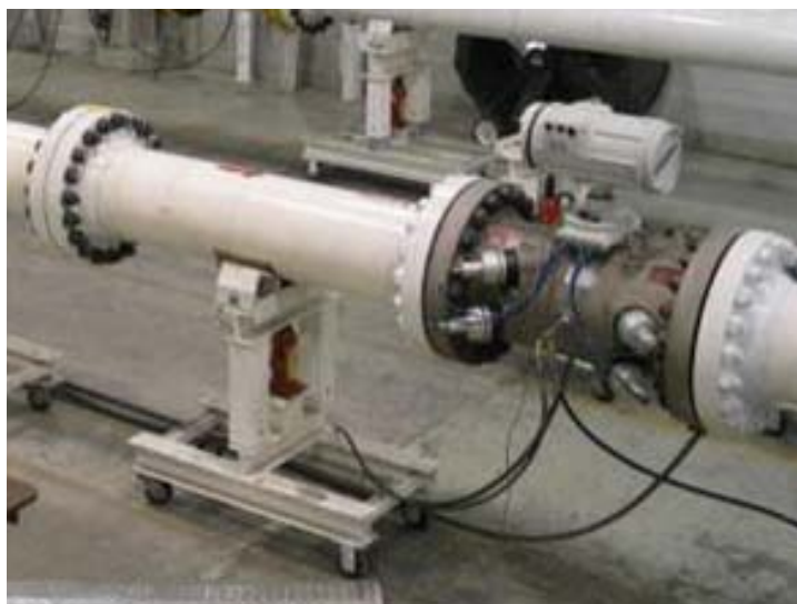
Figure 1. Photograph of the flowmeter installed in the pipeline
