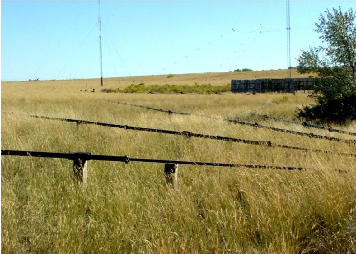
Figure 1.13. Transmitter to antenna transmission lines at WWV.
