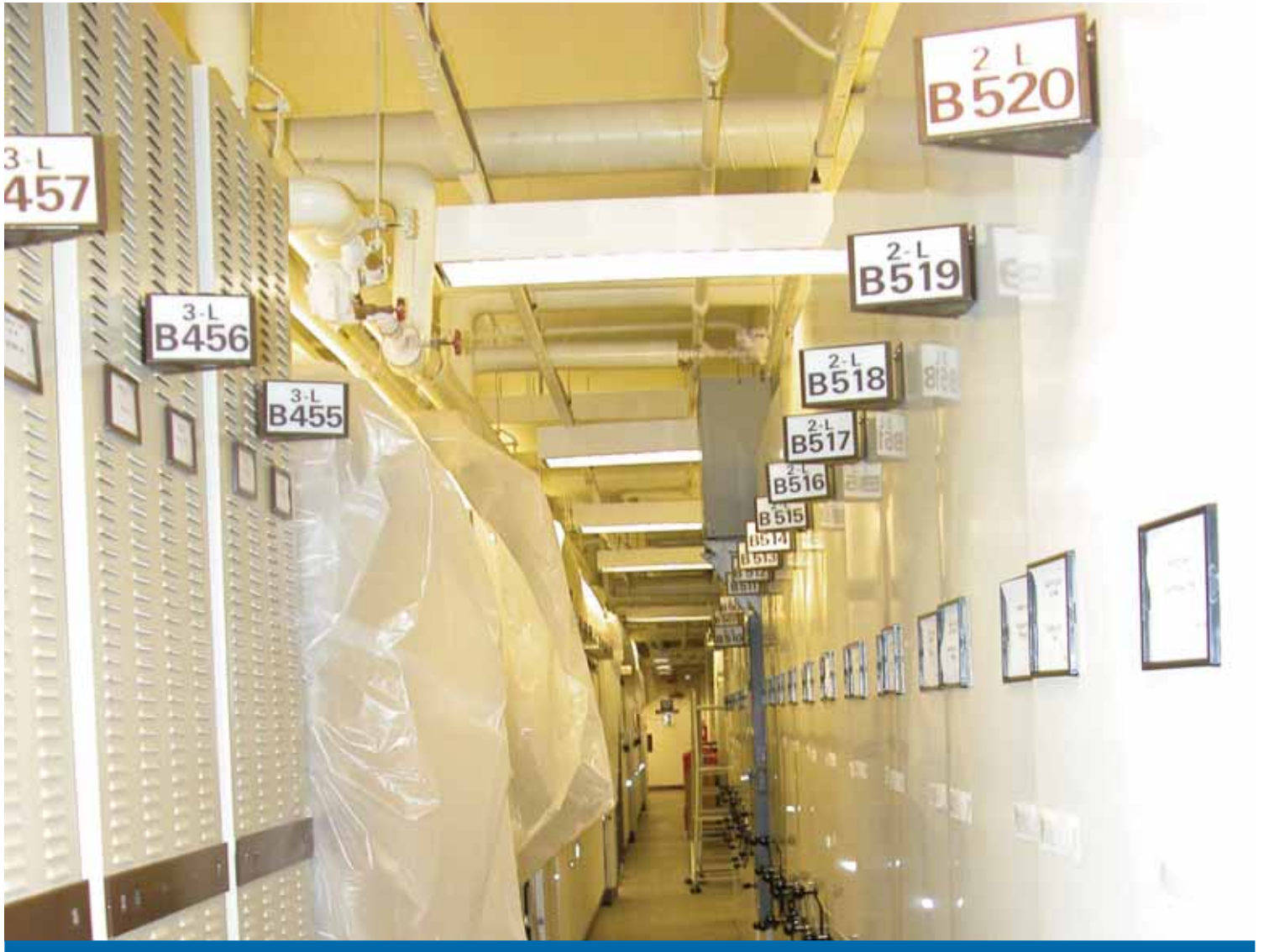
Law Library sub-basement stack area that was affected by a series of water leaks. These books were covered with plastic to avoid further damage from the water.
