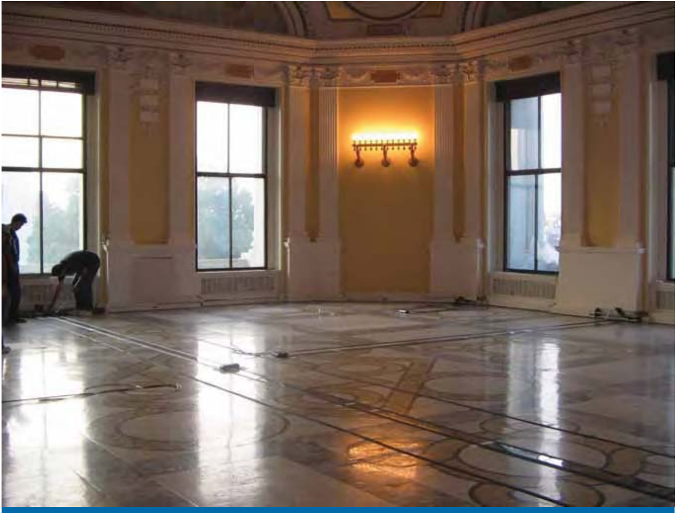
Architect of the Capitol Electrical Shop staff installing electrical flatwire on marble for the European Reading Room relocation
