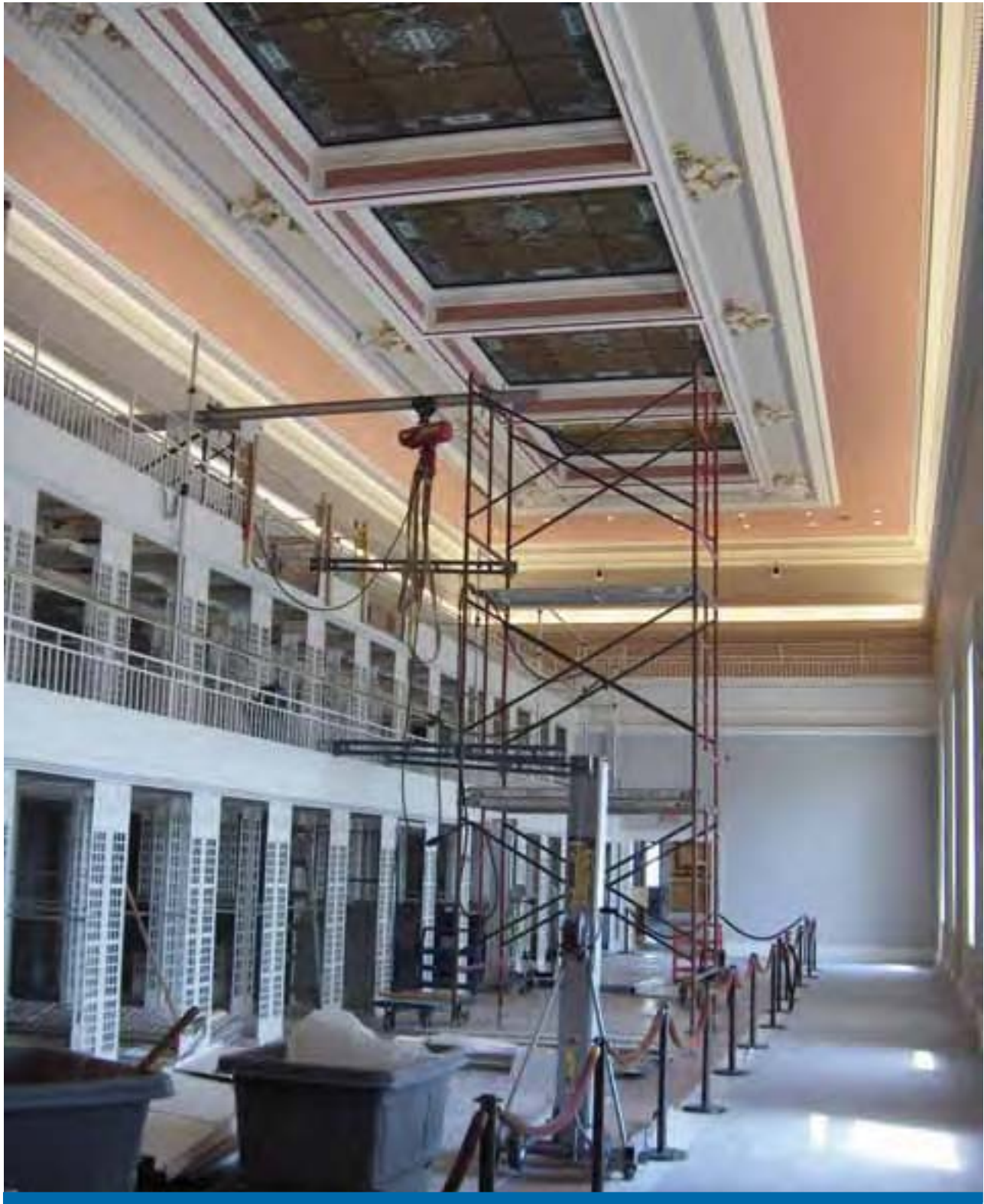
In progress removal of shelving and mezzanine stairs in Northeast curtain, LJ-230. Photo by Karen Bland
