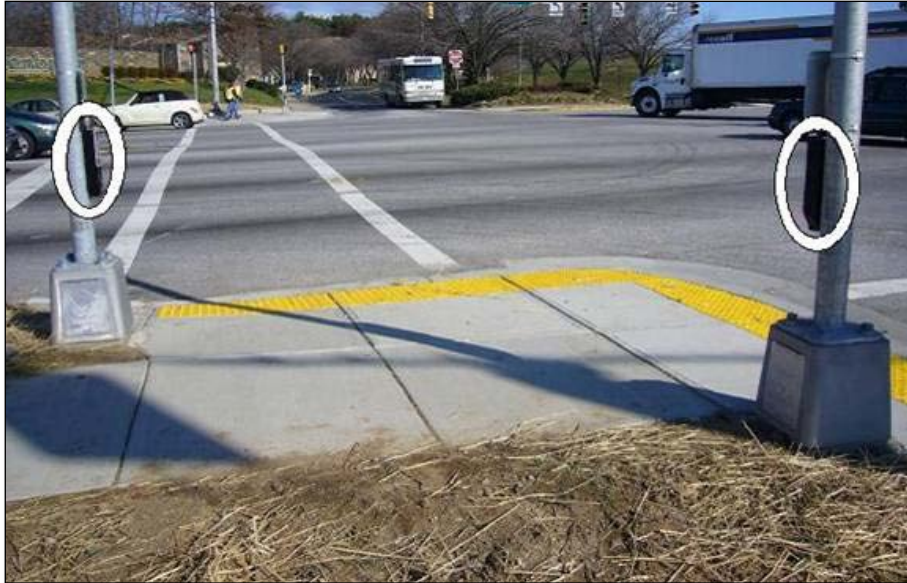
Figure 4: Installation of APS on two separated poles, aligned with crosswalk lines (APS devices circled)
