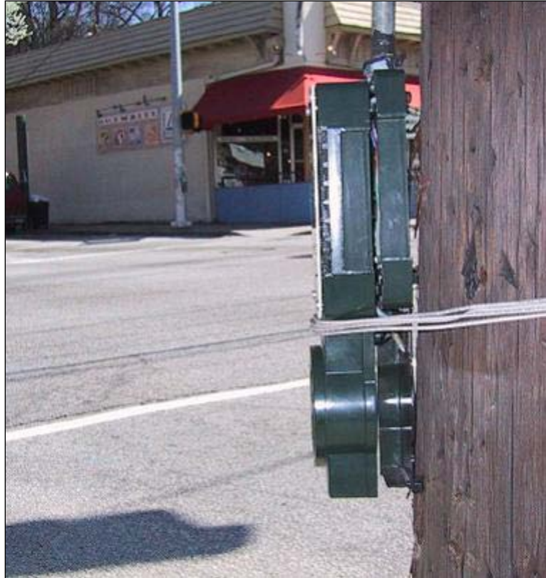
Figure 11: APS that was damaged in a crash and temporarily reinstated with wire.
