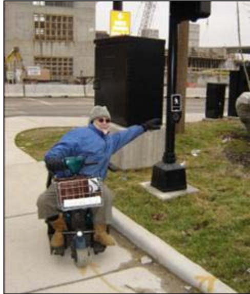
Figure 12: In this new construction, APS is located too far from the sidewalk to be reached by a user of a wheelchair or scooter.
