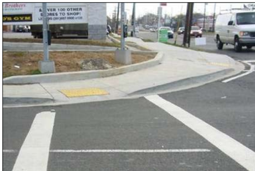
Figure 18: APS and curb ramps that were not installed as designed.
