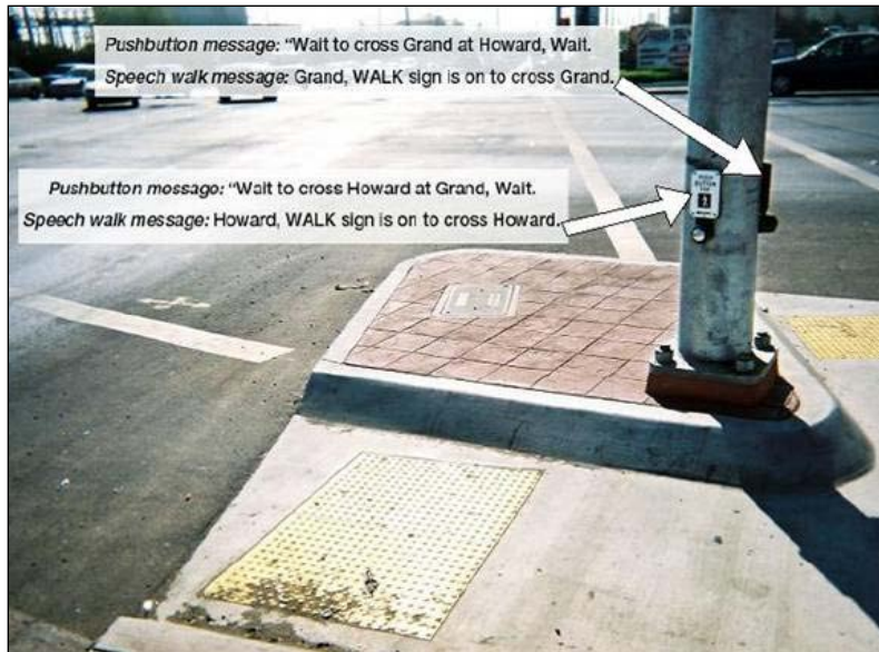
Figure 6: Example of pushbutton information messages and speech walk messages, if two APS must be mounted on the same pole Alterations only.
