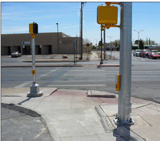
Figure 7: Installation where APS are installed in wrong locations; both are too far from street they control and will be heard as closer to the other street.
