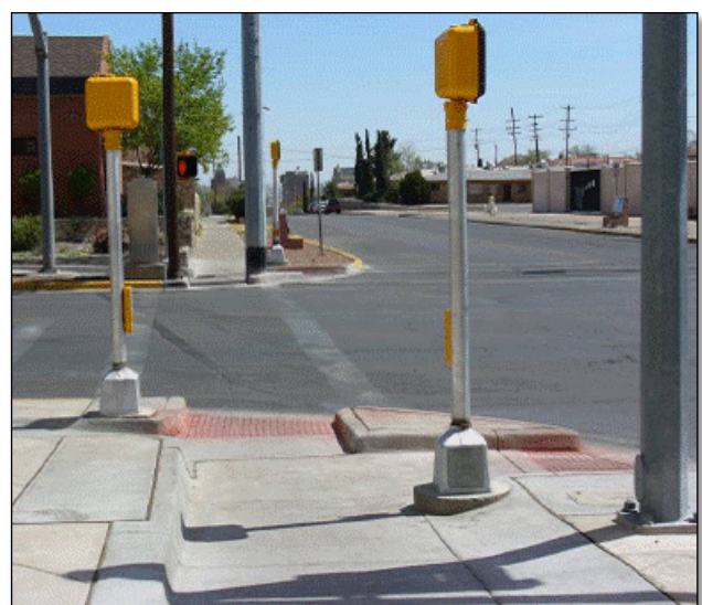
Figure 8: Installation where APS are installed in correct locations in relation to crosswalks.
