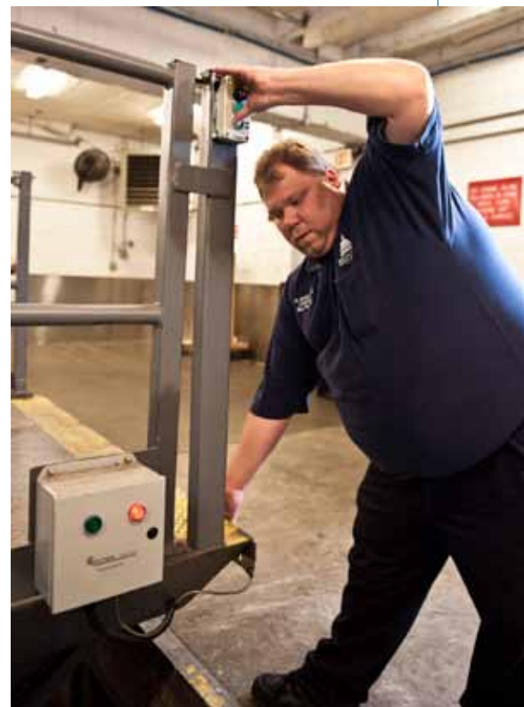
Industrial Mechanic Equipment Leader Brian Bradley tests the pressure switch on the loading dock leveler in the Rayburn Building.
