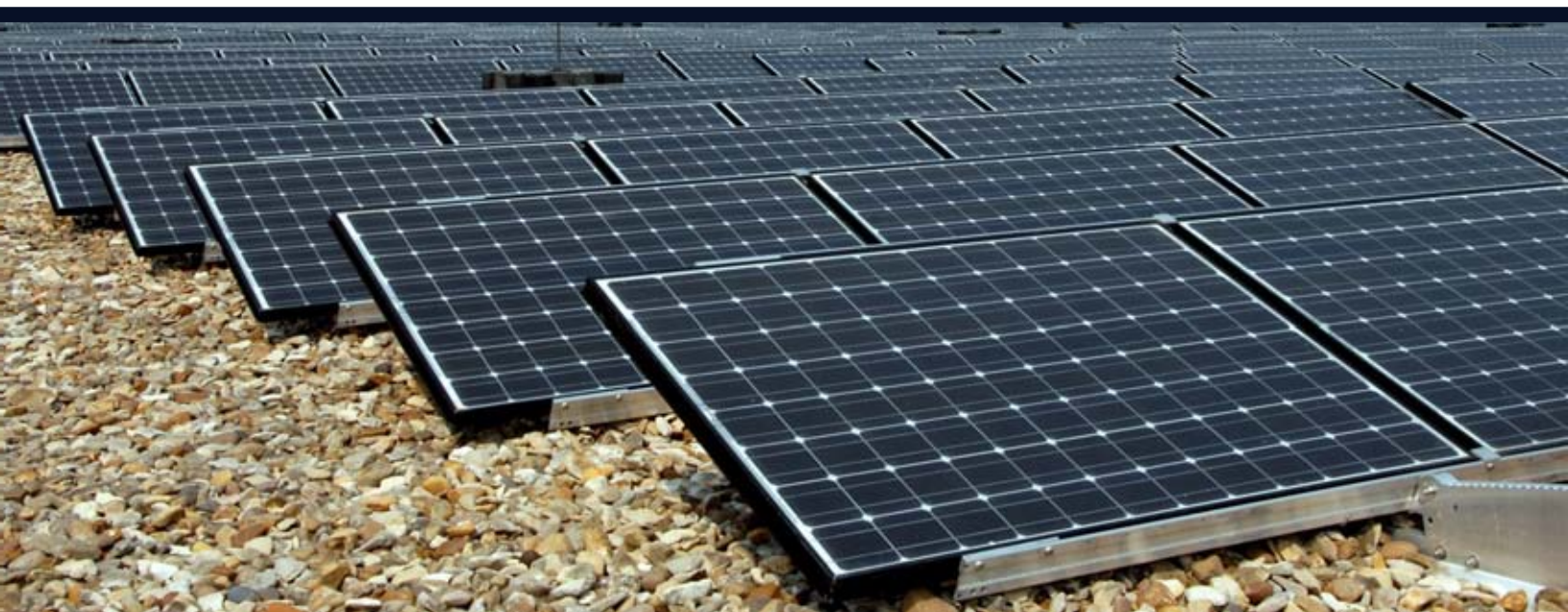
Solar PV pilot program at Dallas VA Medical Center
