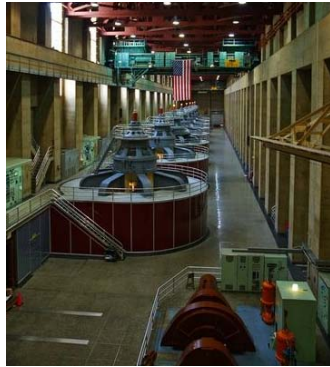
Electric Power Generation
