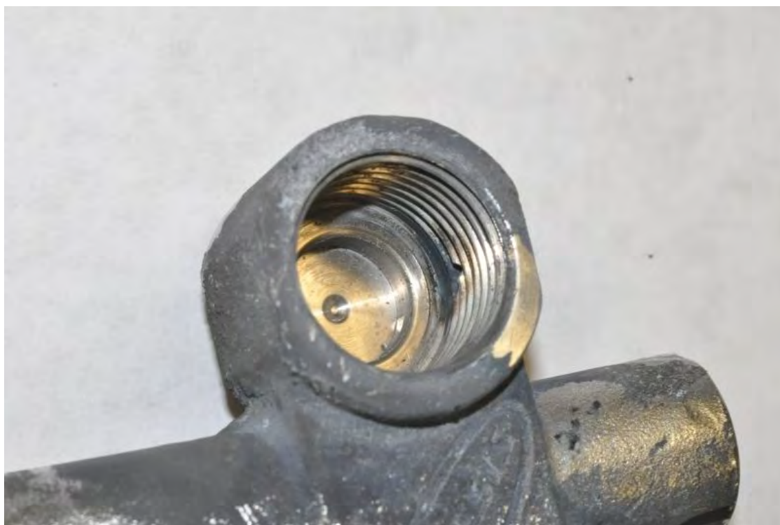
Figure 19. View of the incident valve high pressure regulator port showing discoloration sooting around the vent.
