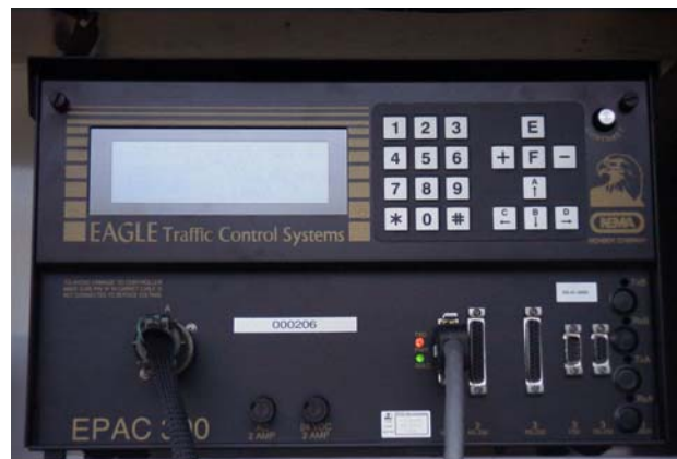
FIGURE 35. EAGLE EPAC300 CONTROLLER SHOWING KEYPAD FOR ENTERING INFORMATION AND WIRING CONNECTIONS.
