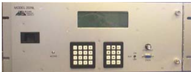
FIGURE 44. MCCAIN 2070 CONTROLLER SHOWING KEYPAD FOR ENTERING INFORMATION AND WIRING CONNECTIONS.
