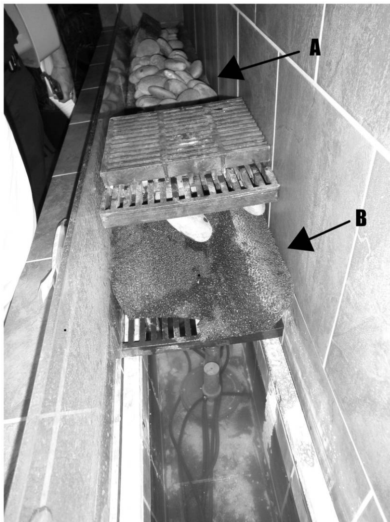
FIGURE 2. Internal view of the water wall-type fountain, showing a bed of decorative rocks that rested on a spongelike foam material. Arrow A points to the decorative rocks in the fountain, and arrow B points to the location of the foam material that was placed in the fountain to prevent splashing. A color version of this figure is available in the online edition.
