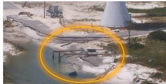
Figure 18. Underwater Cable Crossing Exposed
