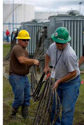
Figure 12. Portable Generator Cabling
