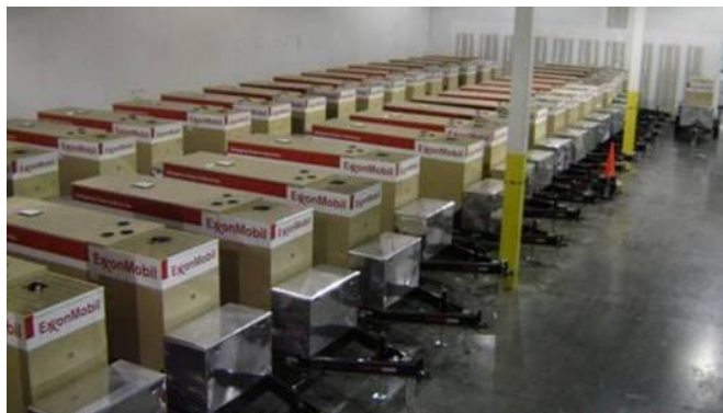
Figure 14. Portable Generators for Retail Stations
