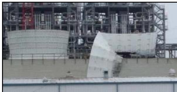
Figure 5. Damaged Cooling Tower Shroud
