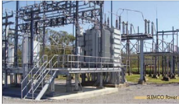
Figure 20. Elevated Substation in Vermilion Parish, Louisiana
