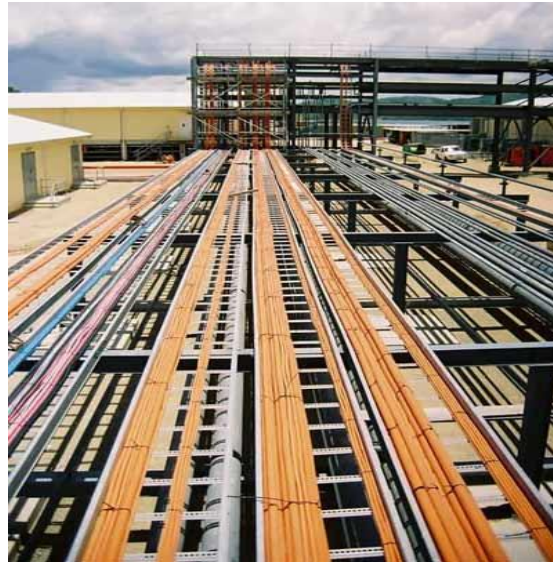
Figure 7. Cable Tray in a Refinery
