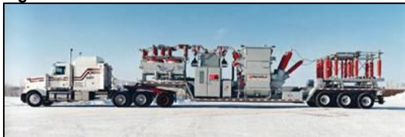
Figure 23. Trailer-Mounted Mobile Substation
