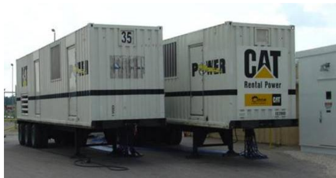
Figure 11. Large Mobile Generators
