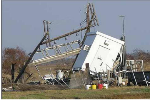
Figure 19. Substation Damage in Vermilion Parish, Louisiana
