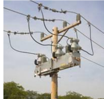
Figure 29. Installed IntelliRupter Recloser
