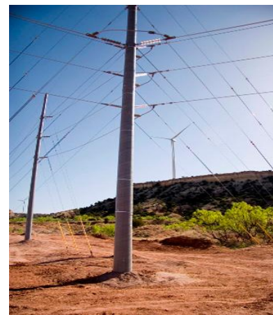
Figure 26. Composite Distribution Pole
