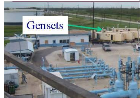
Figure 13. Portable Generators in Texas
