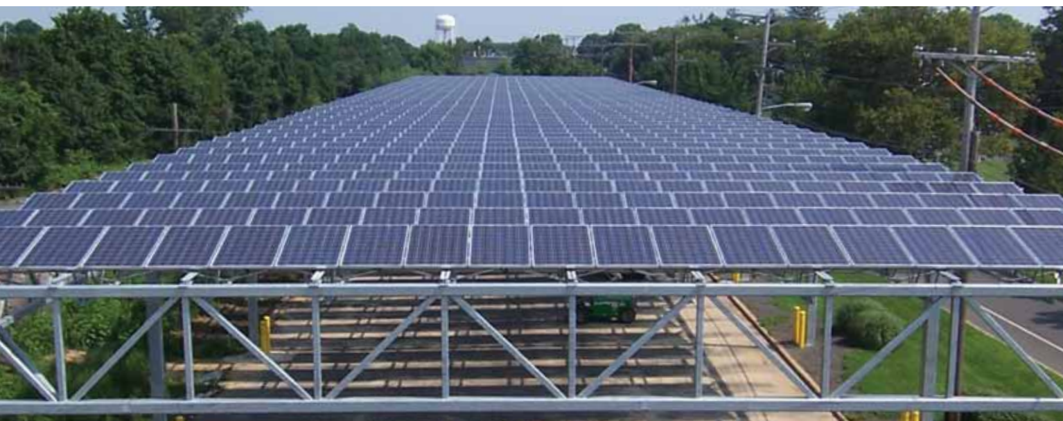
Today, renewable energy makes up 10 percent of the New Jersey Army National Guard's total energy consumption. The goal is to increase that figure to 50 percent by 2020. Here, a carport installation at the National Training Facility Headquarters at Sea Girt. (Photo courtesy of NJ-ARNG)
