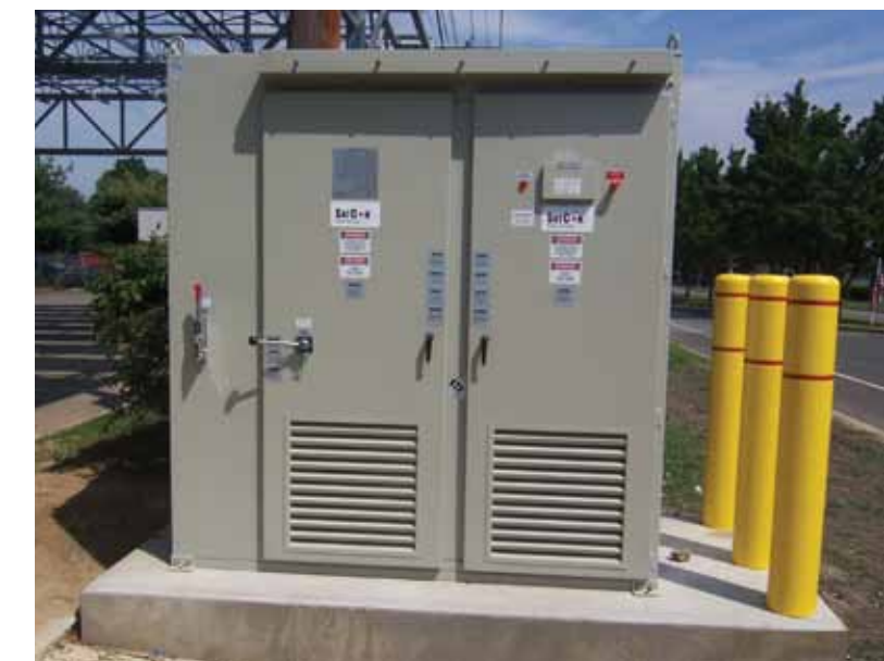
The direct current (DC) output from the photovoltaic modules at Sea Girt is converted by inverters into usable alternating current (AC) electricity that is then fed into the facility's electrical distribution system. (Photo courtesy of NJ-ARNG)
