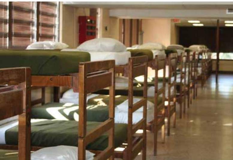
The 40 to 50-year old buildings that house the Regional Training Institute at Camp Minden, Louisiana are plagued with failing sheet rock, leaky plumbing systems, and cracked floors. The lack of adequately-sized classrooms makes meeting accreditation requirements difficult. The existing administrative and classroom space is less than 40 percent of the space authorized. There are also an inadequate number of billets for students, and most billets have group restrooms and showers.
