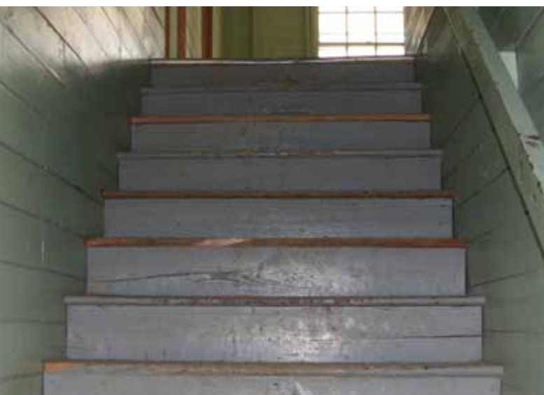
Above left: A typical stairwell in a World War II-era barracks at Fort Indiantown Gap, Pennsylvania. Above right: A cracking floor at Fort Chaffee, Arkansas.
