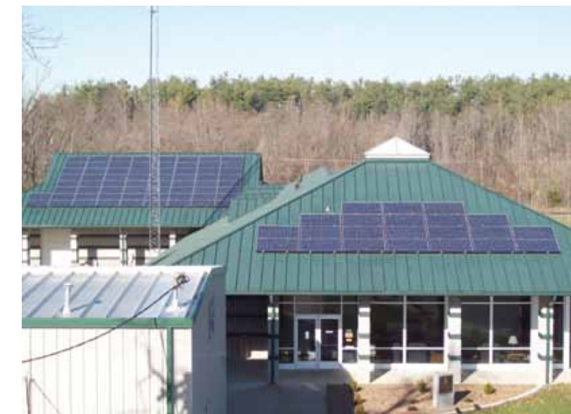
At the Wendell H. Ford Regional Training Center in Greenville, Kentucky, ARRA funds financed a $553,500, 84 kW photovoltaic system made up of 400 solar panels, which will produce approximately 100,000 kW hours of renewable green energy a year. The 400 solar panels are tied to the local grid, and any excess power will flow back onto the grid, running the facility power meter backwards and creating a credit.
