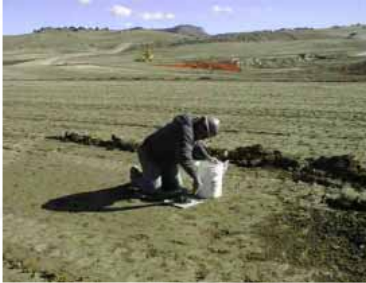
Quality control test on mill tailings cover at L-Bar site in New Mexico
