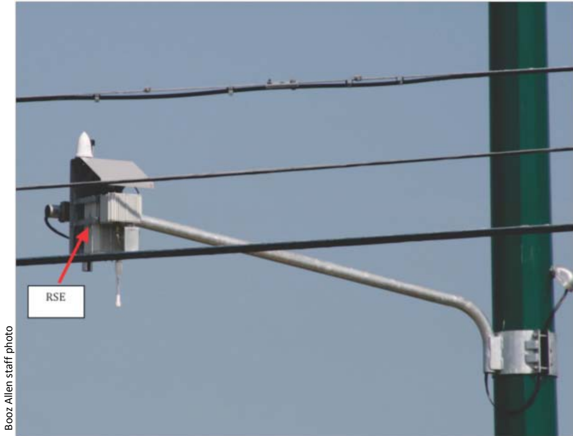
Figure 2-50: Typical RSE Field Installation
