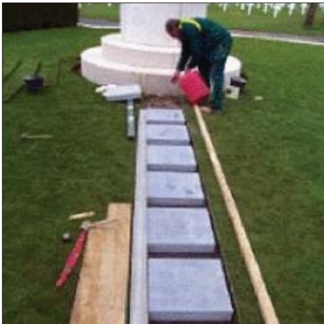
A new walkway from the memorial to the flagpole is installed at St. Mihiel Cemetery
