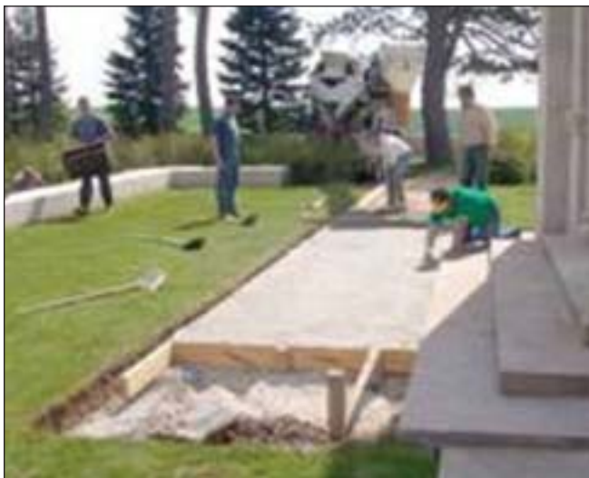
A ramp is installed to provide handicapped access to the Meuse-Argonne Cemetery chapel
