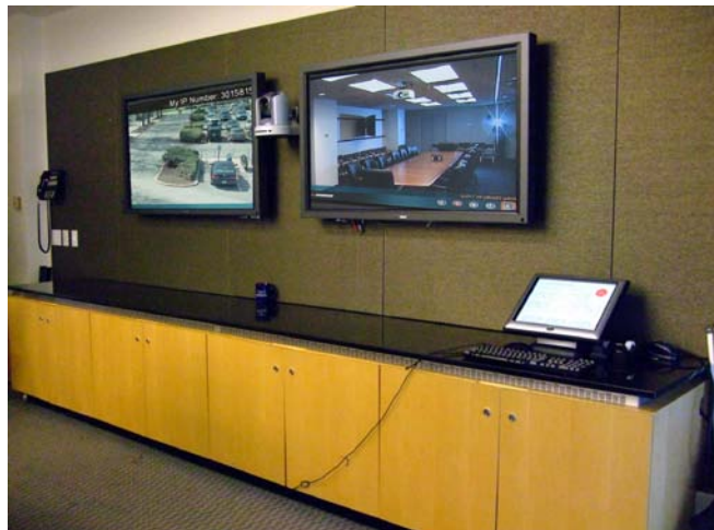
[Caption: This room has twin wall-mounted plasma screens above the hardware cabinets. The touch-panel is on the counter at the far right.]
