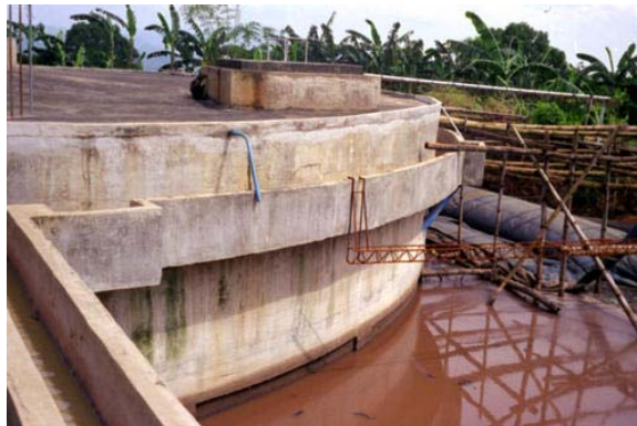
Figure 7. Concrete digester on a hog farm. Source: NREL PIX.
