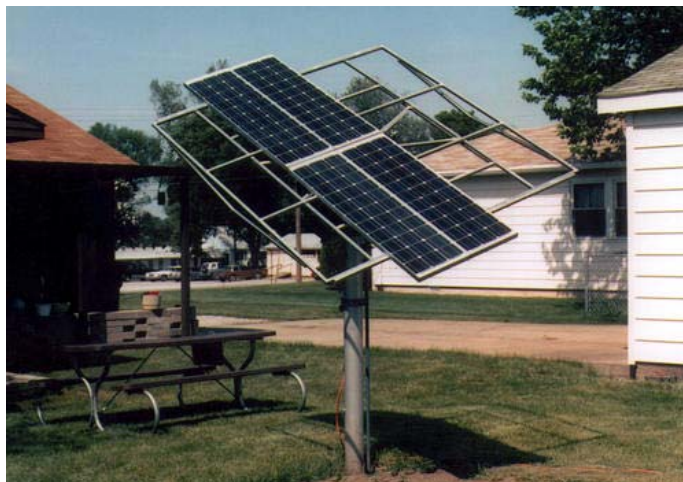
Figure 17. Modern photovoltaic (PV) array. Source: NREL PIX.
