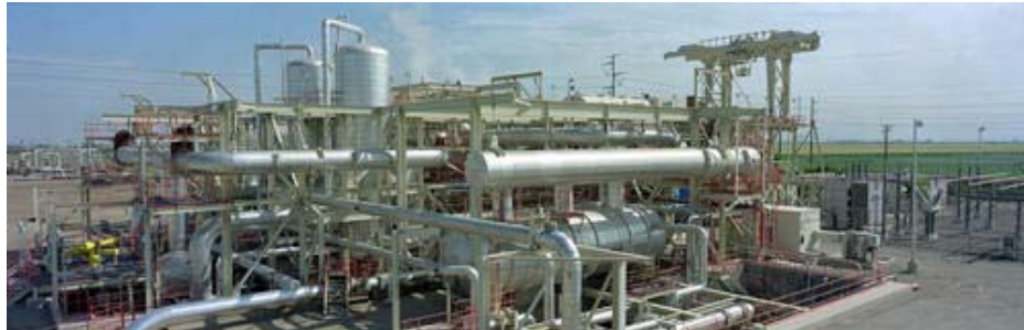
Figure 35. Dual flash geothermal power plant. Source: NREL PIX.
