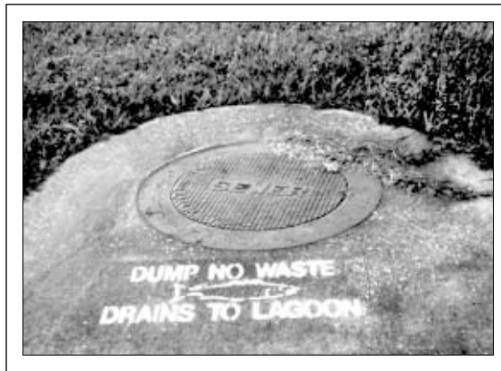
Clearly label stormwater sewers to discourage dumping of hazardous wastes.
