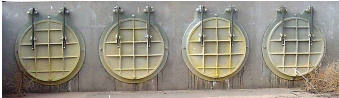
Figure 2.64 ACCEPTABLE flap gates in earthen levee. (KS)
