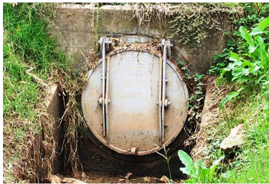
Figure 2.65 UNACCEPTABLE vegetation around flap gates in earthen levee. (OK)
