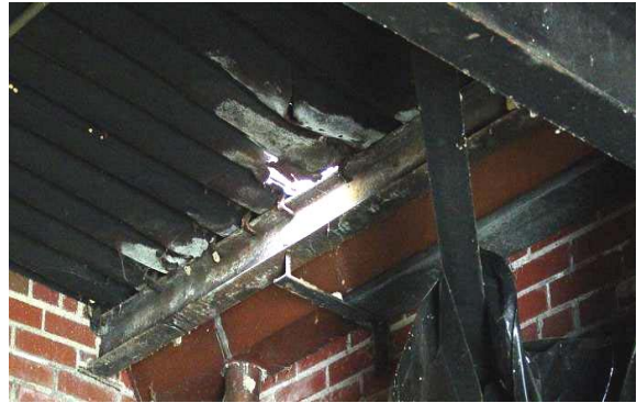
Figure 2.67 Hole in roof of pumping station. (IL)
