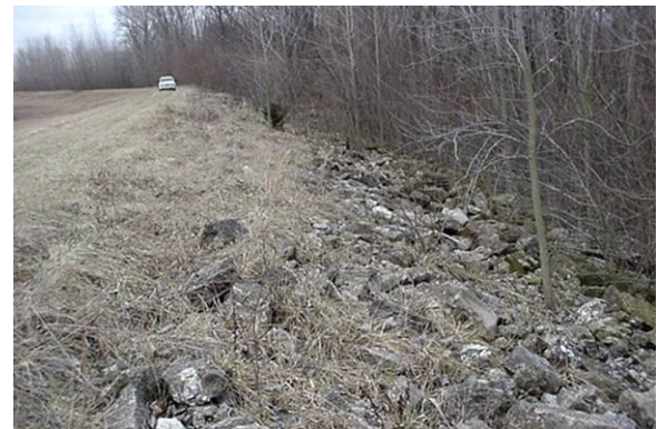
Figure 2.28 UNACCEPTABLE. Tree and sapling growth is well established within the riprap protection on an earthen levee. This overgrowth must be removed. (MO)
