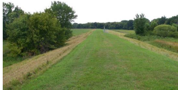
Figure 2.31 UNACCEPTABLE. Levee is mowed but trees and longer grasses within levee easement area. Trees are greater than 2" in diameter. (MN)
