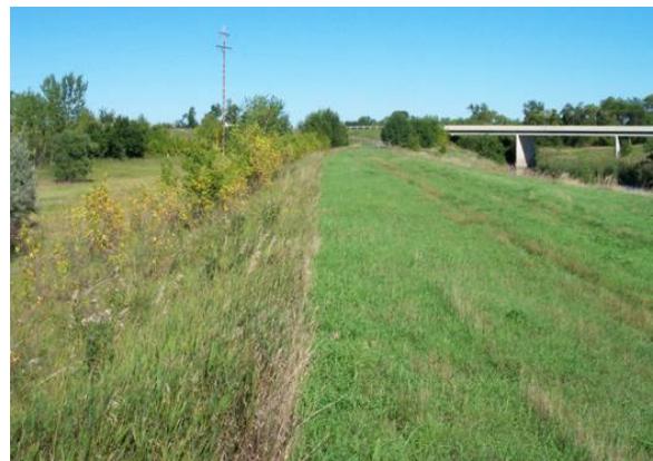
Figure 2.32 UNACCEPTABLE long grasses and trees on levee side slopes. (ND)
