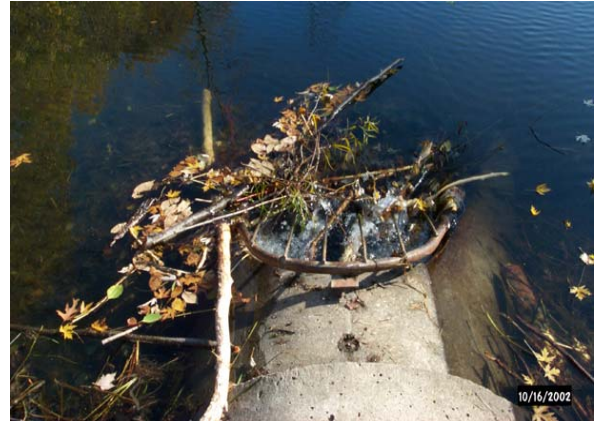
Figure 2.22 Beavers attempting to block the culvert passing through a gated embankment. (MN)
