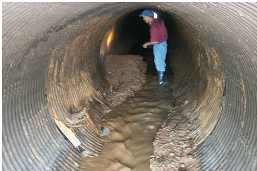
Figure 2.61 UNACCEPTABLE, Failing corrugated metal pipe. DO NOT WALK INTO A FAILING CULVERT LIKE THIS. This section has actually separated, allowing the surrounding soil to enter the pipe and the overburden to collapse. This sponsor was denied rehabilitation assistance due to this maintenance deficiency.
