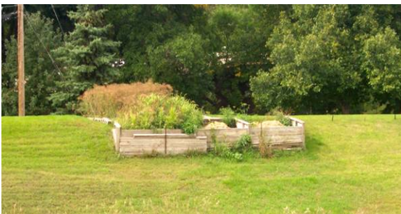
Figure 2.13 UNACCEPTABLE encroachment. Gardens and compost bins located on levee crest and riverward slope. (ND)
