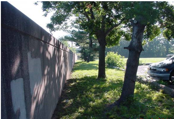
Figure 2.51 UNACCEPTABLE. Trees growing too close to floodwall. (KY)
