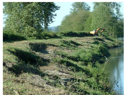
Figure 2.3 Slope failure on bank protection project. (WA)
