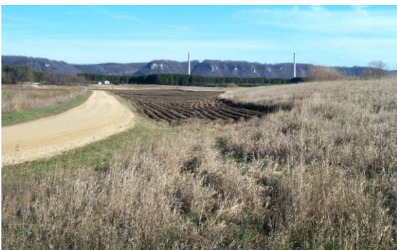
Figure 2.6 UNACCEPTABLE levee encroachments. This landowner tilled near one third of the way up the landward levee slope. (MN)
