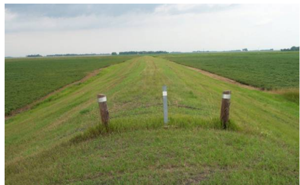
Figure 2.5 MINIMALLY ACCEPTABLE. Field encroaches on levee easement. The landowner has tilled the soil right to toe of the levee, and was requested to stay back at least 10 feet. (ND)
