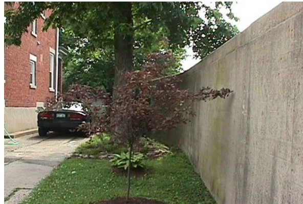
Figure 2.52 UNACCEPTABLE. Trees growing too close to floodwall. (KY)
