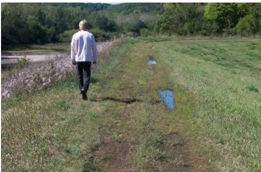
Figure 2.38 MINIMALLY ACCEPTABLE ponded water along a levee crest. (MN)
