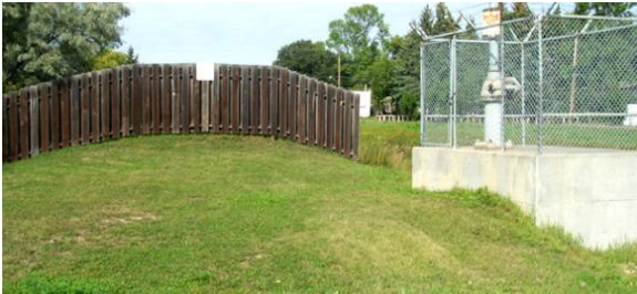
Figure 2.11 UNACCEPTABLE encroachment. Residential and rural fences crossing the levee. (ND)
