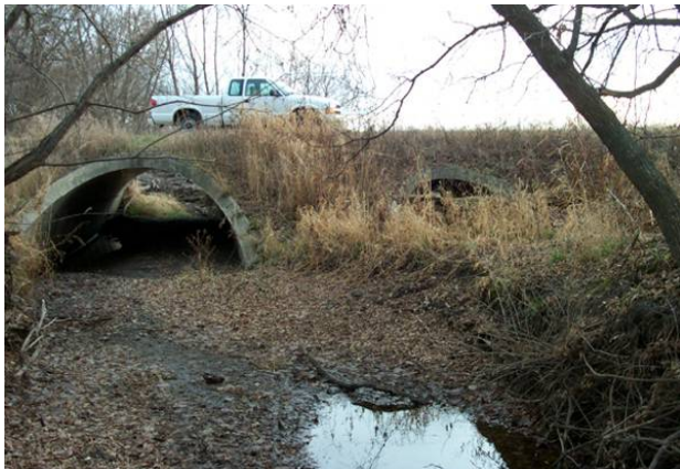
Figure 2.59 The culvert on the left is Minimally Acceptable with sediment accumulation within the culvert. The culvert on the right is totally unacceptable with 2/3 of its flow capacity reduced by sediment and debris. This project was rated as UNACCEPTABLE because of the reduced flow capacity of the culverts. (MN)
