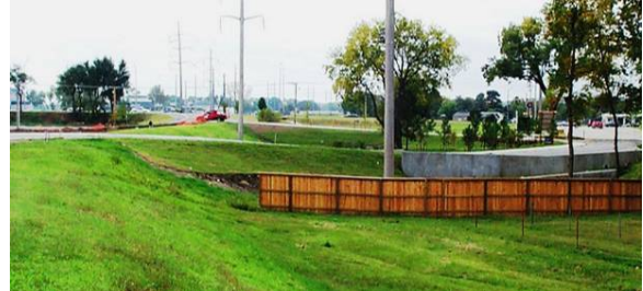
Figure 2.12 UNACCEPTABLE, unapproved encroachment on levee easement (fencing). (OK)
