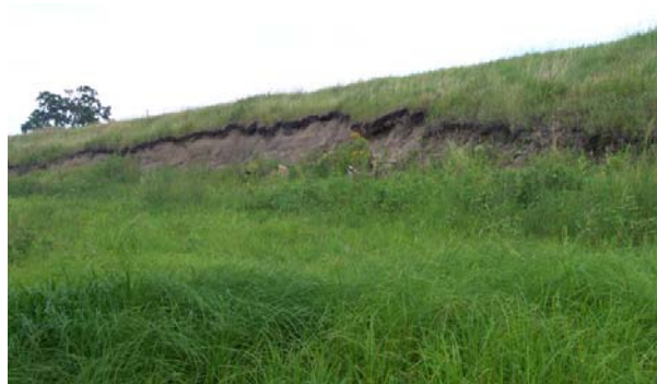
Figure 2.17 UNACCEPTABLE earthen embankment failure. (MN)
