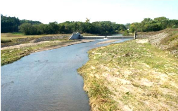
Figure 2.70 UNACCEPTABLE channel shoaling below a control structure. The original channel bottom extended all the way to the riprapped banks. There is an estimated 2-3 feet of sediment in the channel, mostly from upstream field erosion and highway construction. (MN)
