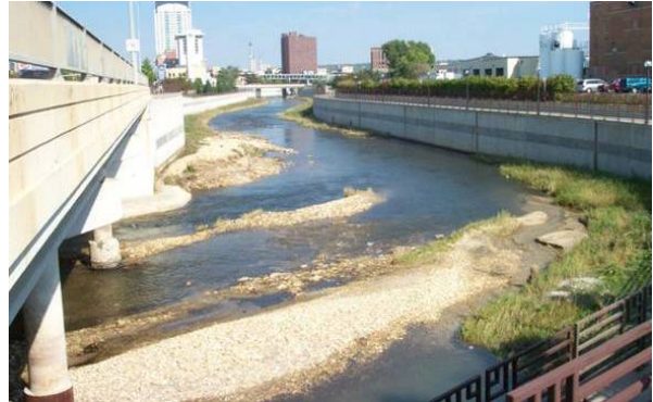
Figure 2.71 MINIMALLY ACCEPTABLE shoaling within a concrete lined channel. (MN)
