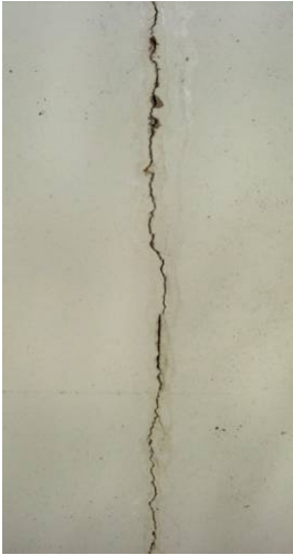
Figure 2.43 MINIMALLY ACCEPTABLE 1/8 th inch crack extends through concrete floodwall and needs to be sealed to prevent further damage. (MN)
