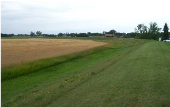
Figure 2.4 ACCEPTABLE. Landowner has not encroached on levee easement area and has stayed back 10 - 15 feet. (MN)
