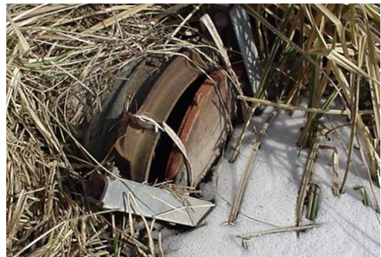
Figure 2.66 UNACCEPTABLE flap gate in earthen levee. (Broken hinge and vegetation growth.) (MO)
