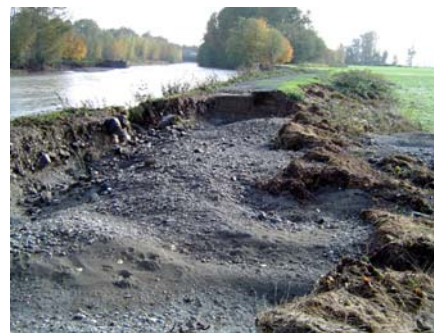
Figure 2.2 Flood damage. (WA)
