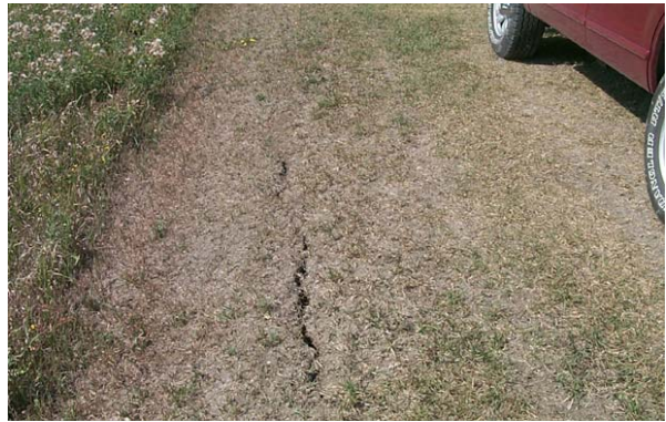
Figure 2.33 ACCEPTABLE cracking in clay levee with shrinkage cracking caused by dry conditions. (MN)
