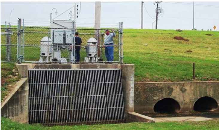
Figure 2.68 Pump station beside earthen levee. (OK)
