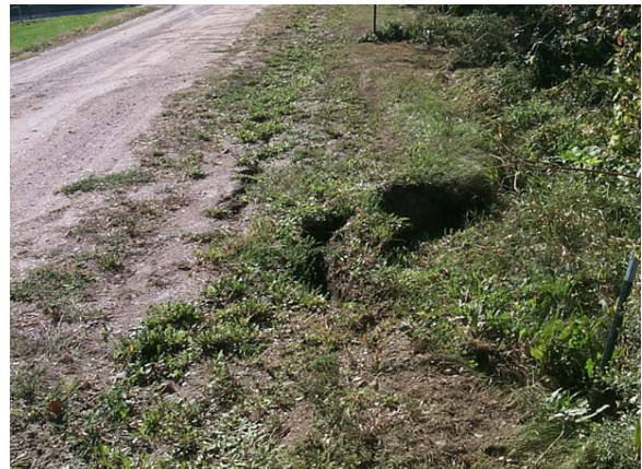
Figure 2.35 UNACCEPTABLE embankment cracking and slope failure. This photo shows what started out as cracking along the crest of the embankment and quickly developed into a slope failure. All cracking located on a levee or riverbank must be closely monitored. (MN)
