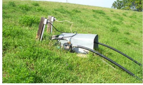
Figure 2.8 UNACCEPTABLE encroachment. Piping for lawn irrigation system drilled through levee without approval. (ND)
