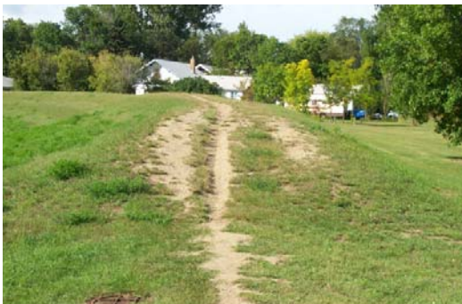
Figure 2.36 MINIMALLY ACCEPTABLE levee rutting caused by pedestrian and bicycle traffic. (ND)
