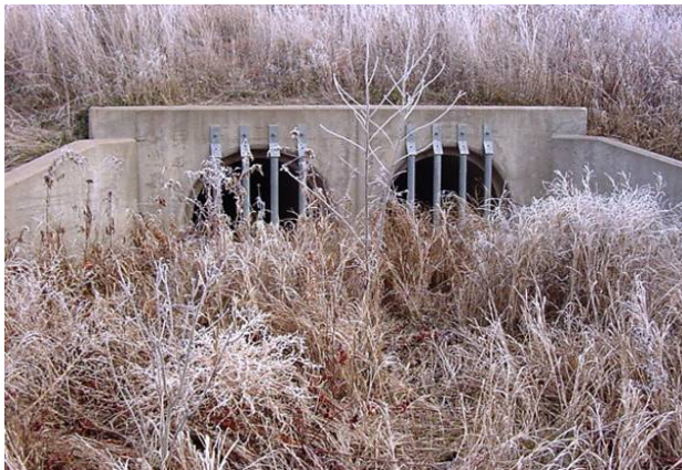
Figure 2.60 MINIMALLY ACCEPTABLE, vegetation blocking the concrete culvert must be removed. (KS)
