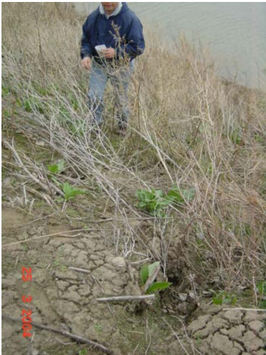
Figure 2.34 UNACCEPTABLE cracking with landside pooling, Whitehead Levee Project, (IA)
