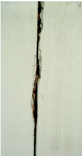
Figure 2.45 UNACCEPTABLE exposed rebar. Monolith joint separation with exterior spalling along the joint and interior spalling in the area of the rebar. (MN)
