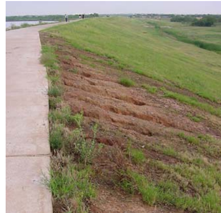
Figure 2.1 UNACCEPTABLE erosion of levee slope. (TX)
