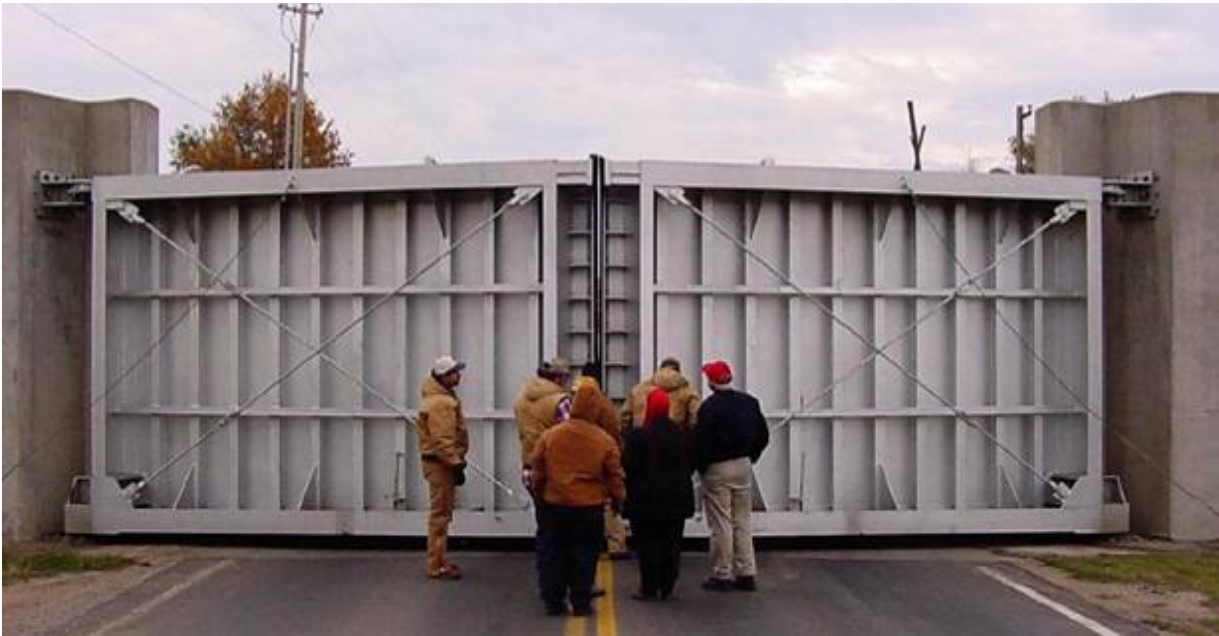
Figure 2.42 ACCEPTABLE floodgate in a levee. (KS)
