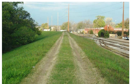
Figure 2.39 UNACCEPTABLE rutting in levee. (OK)
