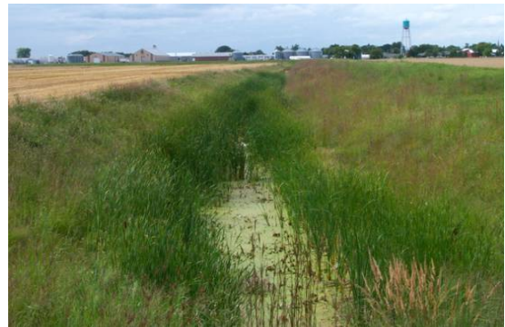
Figure 2.55 MINIMALLY ACCEPTABLE vegetation (cat tails and bull rushes) in interior drainage ditch. (MN)
