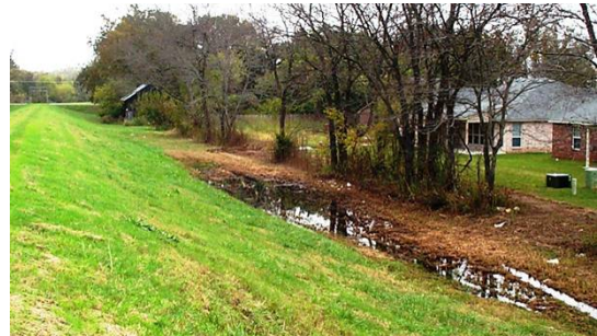
Figure 2.53 UNACCEPTABLE interior drainage at the toe of an earthen levee. (OK)
