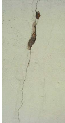
Figure 2.44 MINIMALLY ACCEPTABLE Vertical floodwall crack with spalling. The rating for this particular crack is Minimally Acceptable because the crack is still tight but there is some spalling occurring as well. (MN)
