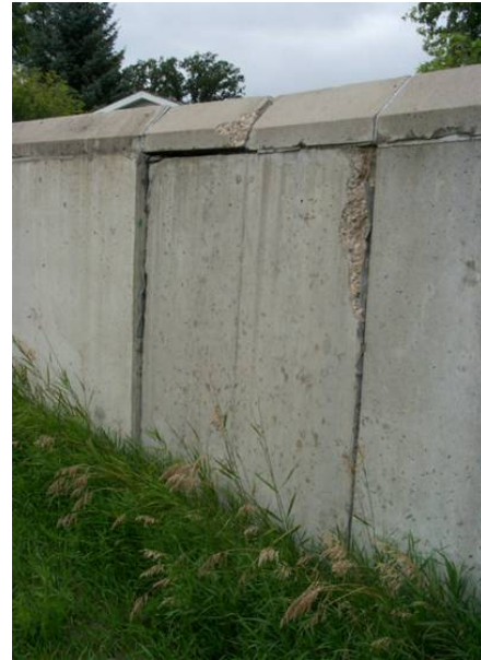
Figure 2.49 UNACCEPTABLE monolith movement in floodwall. The monolith shown in the photo has tilted about 6 inches riverward as well a vertically. Note the movement when compared to the adjoining monolith and the top cap. As the monolith moved considerable spalling has occurred along the joint. This project is monitored very closely during flood events. (ND)
