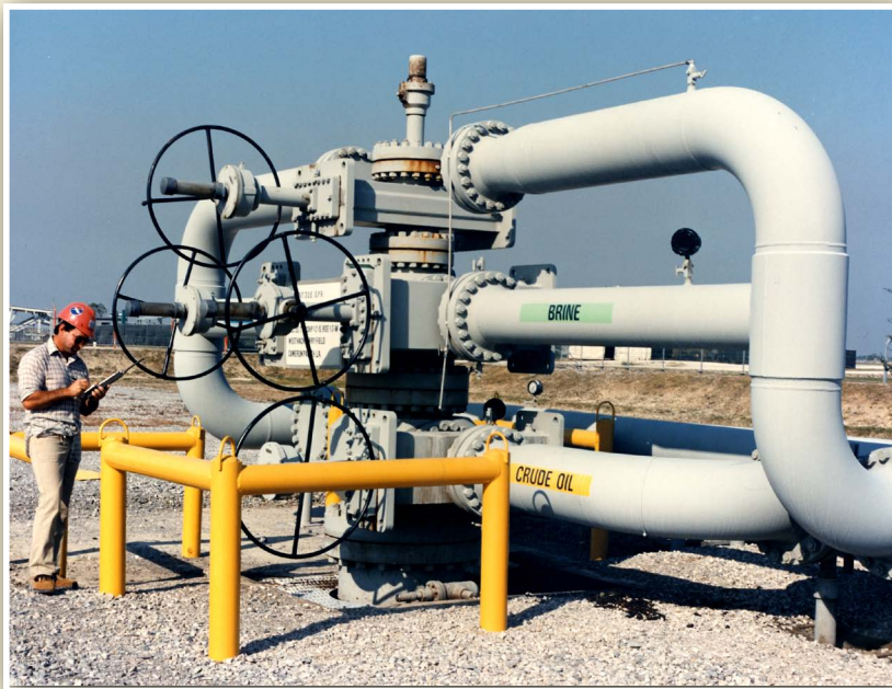
A technician inspects wellhead assembly at the Reserve's West Hackberry site near Lake Charles, LA.
