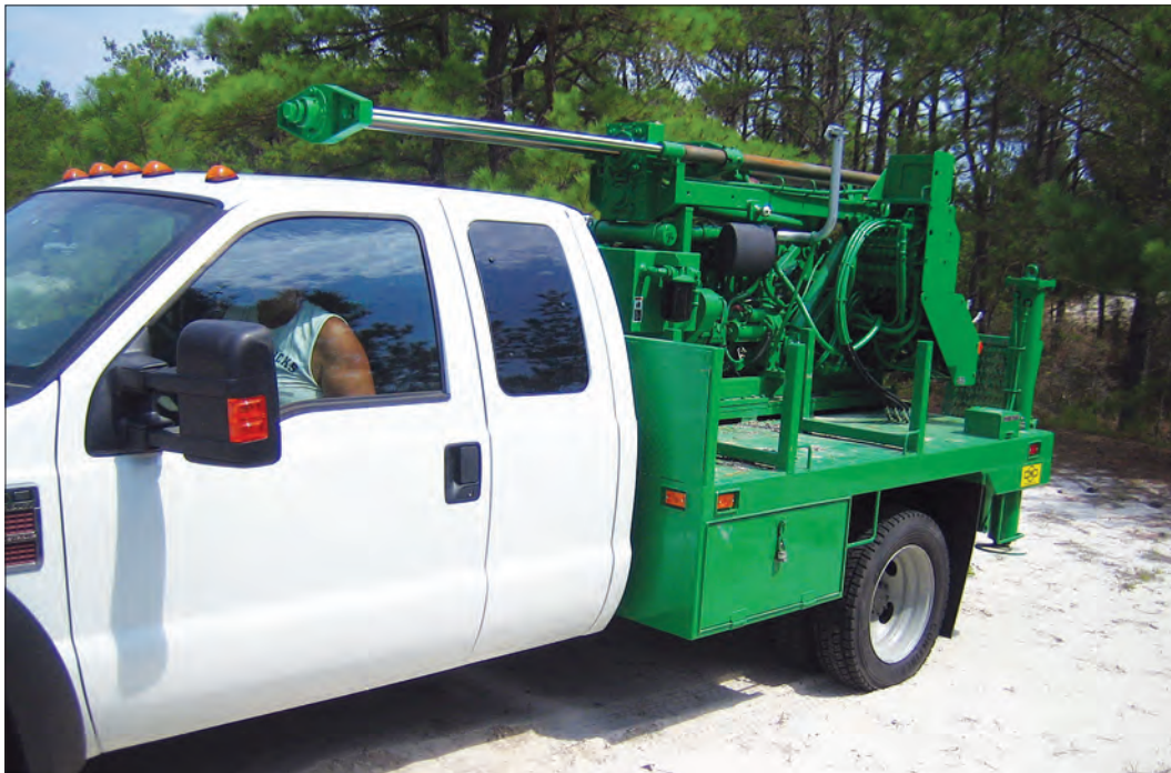
Figure 3. Truck-mounted hollow-stem auger drill rig used for monitoring well installation on Assateague Island National Seashore, Worcester County, Maryland. [Photograph by William Banks, U.S. Geological Survey, Aug. 8, 2010.]
