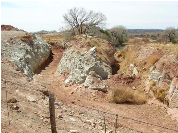
e. Downstream view: New ditch alignment (left) cut July 2008 in response to wash-out of previous channel (right)
