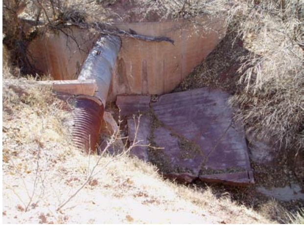
b. Flume 1, erosion around pipe.
