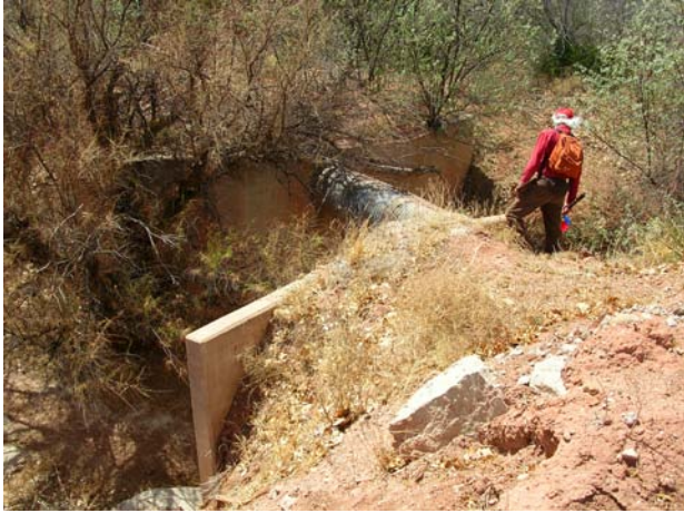
a. Flume 1, erosion around concrete abutment
