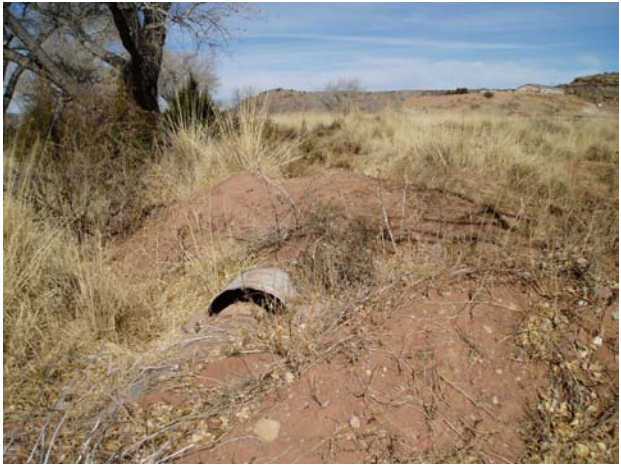
d. Flume 2, gap in existing pipe.
