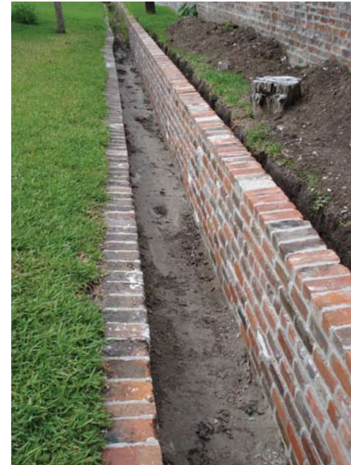
Just like the towers on the left, these historic drainage gutters on Jackson Barracks were carefully restored after sustaining much damage.
