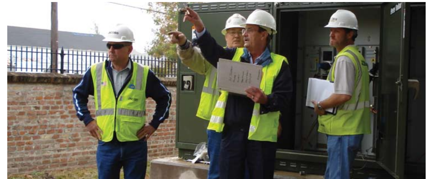
Louisiana Army National Guard inspectors put the new electrical infrastructure through the paces during commissioning. Hurricane Katrina completely destroyed all utilities on Jackson Barracks.
