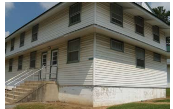
Top: The average age of the Army National Guard’s facilities is over 40 years old. The facilities in the foreground of this aerial photo of Ft. Indiantown Gap, Pennsylvania are WWII vintage facilities. The green metal roofs were installed to protect and preserve the wood barracks. Middle: The interior of a barracks in need of renovation at Ft. Indiantown Gap. Bottom: Barrack exterior at Ft. Indiantown Gap.
