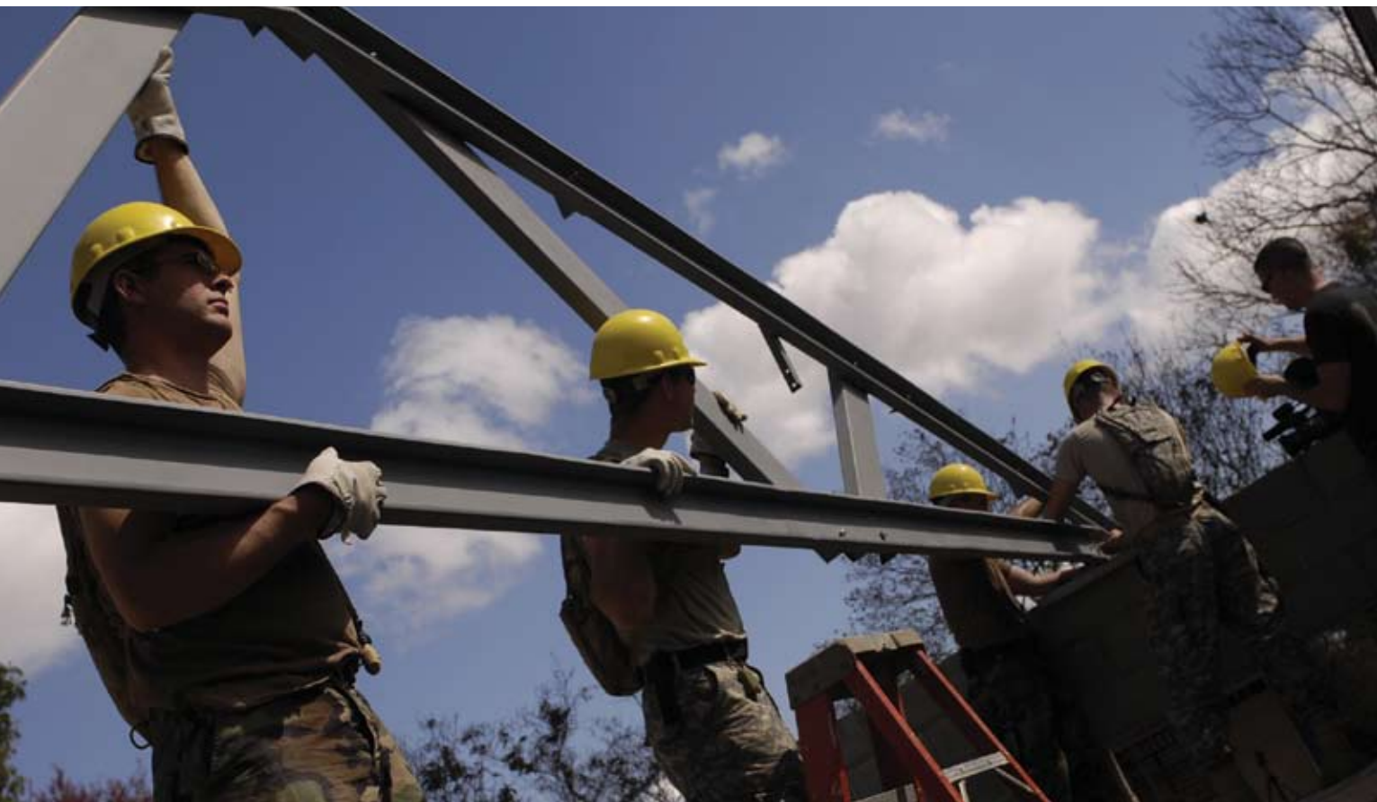
Above and opposite page: Soldiers from the 153rd Engineering Battalion, North Dakota Army National Guard, install rafters at a school. (Photo by Staff Sgt. Jason T. Bailey)
