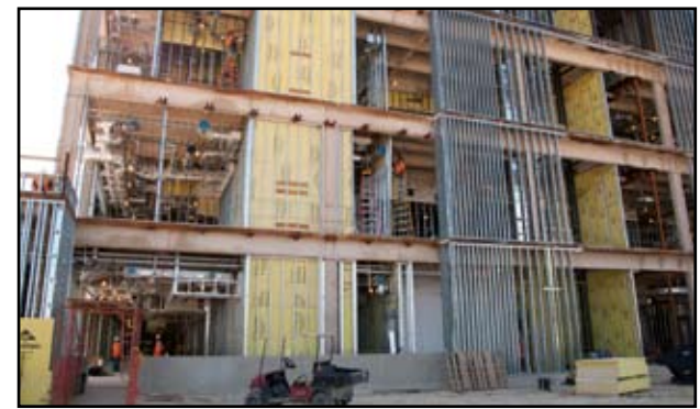
Construction workers install electrical wires and air conditioner ducts in the new Wilford Hall Ambulatory Surgical Center “A” wing on Joint Base San Antonio-Lackland Aug. 28. The wing is part of the first phase of the WHASC construction project, which includes a 1,000-car parking garage and a new energy plant that is nearly 67 percent completed.
