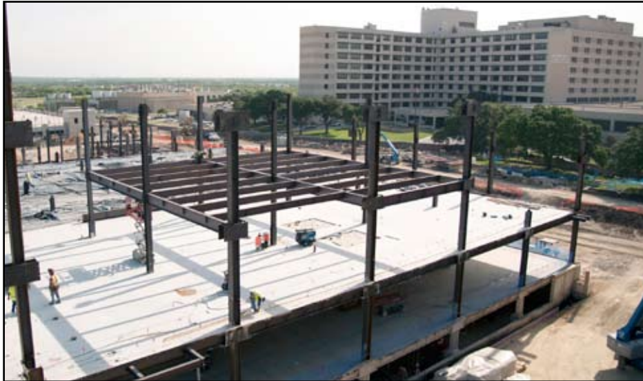
Wilford Hall Ambulatory Surgical Center overlooks the construction of the “B” wing for the new WHASC on Joint Base San Antonio-Lackland, Texas, Aug. 28. This is one of four wings and is part of the second phase of the construction project that is currently 16 percent completed. Between each wing will contain garden spaces that will provide a healing and therapeutic environment for patients.
