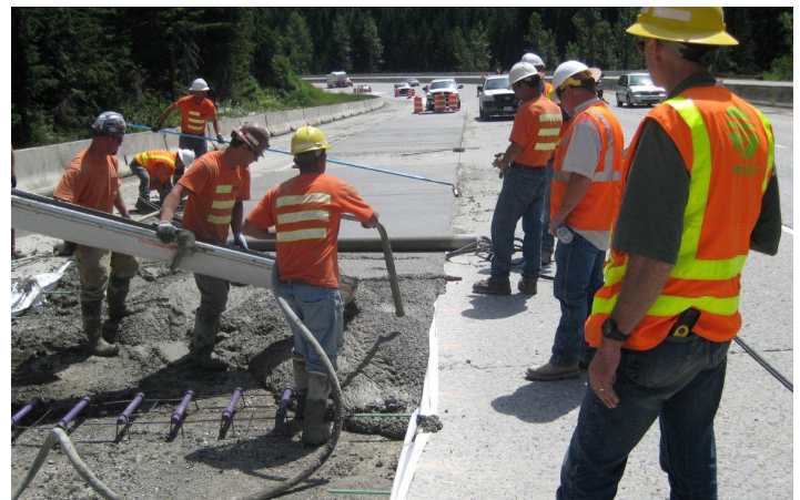
WSDOT and Vetch Construction crews install dowel bars and pave I-90 near Snoqualmie Summit.
