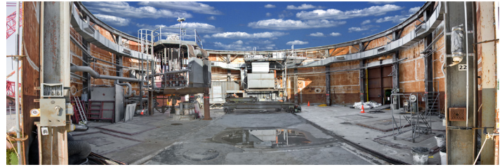
Inside a reactor being decommissioned. (Photo courtesy of Bruce Boulineau)
