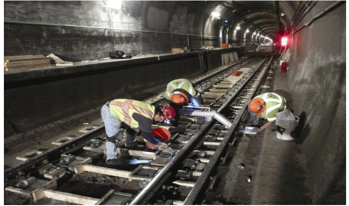
Workers remove old track and replace it with new track. (Photos courtesy of Chicago Transit Authority)
