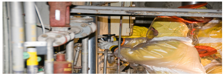
Workers don protective gear for decontamination and decommissioning. (Photo courtesy of Steve Ashe)
