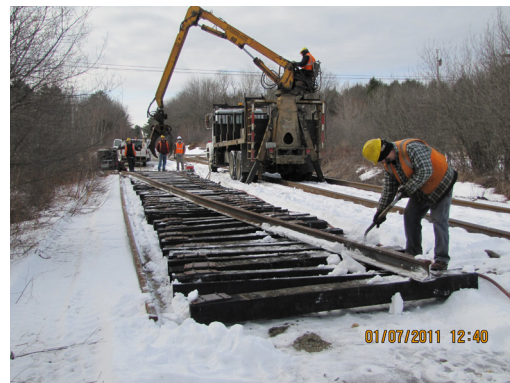
Crews in Maine removing old joint-tethered railroad track to be replaced with new, continuously welded track for high-speed trains.
