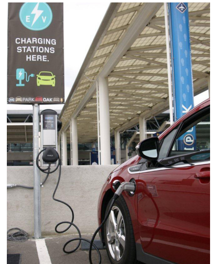
Some charging stations are located in parking garages and lots. (Photo courtesy of Coulomb Technologies.)
