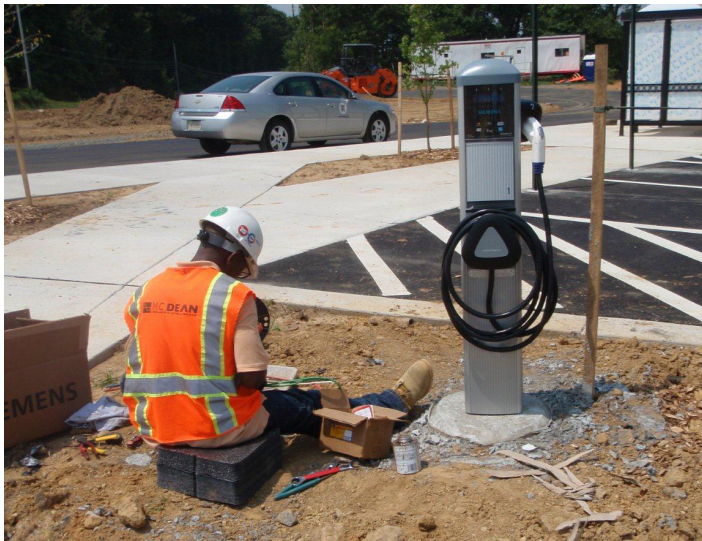
One of five electric vehicle charging stations being installed in Hamilton, VA.
