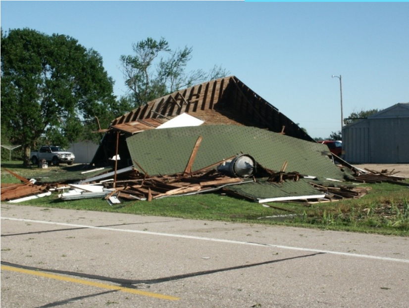
Barn Downed at Hwy 36 and Hwy 275
