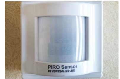
Occupancy sensors in the Courtyard by Marriott San Diego Downtown keep tabs of lighting needs.
