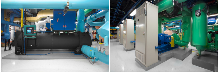
High-efficiency pumps, variable frequency drives, and a new chiller fill the new plant inside the Hines-managed 522 Fifth Avenue building.
