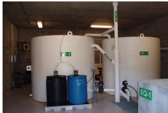
Clarifier at the NETL-Morgantown site
