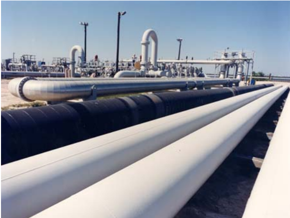
Crude oil pipelines at SPR's Bryan Mound site.
