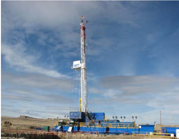
A RMOTC drilling rig located on the 10,000-acre Teapot Dome Oil Field.
