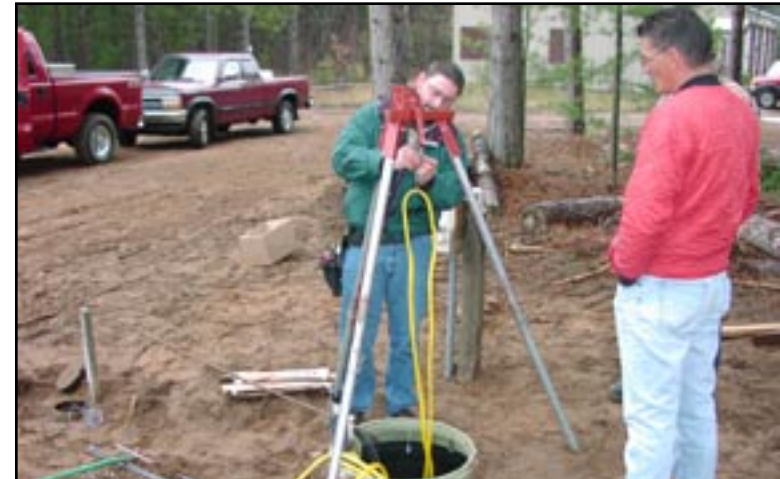
Figure 23: James Valliere, LDF Assistant Operator, and contractor setting up hoist to remove the grinder pump, Lac du Flambeau, MI.
