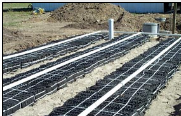
Figure 46: An Eljen in drain leachfield system installed for a new homeowner at Taos Pueblo, New Mexico.
