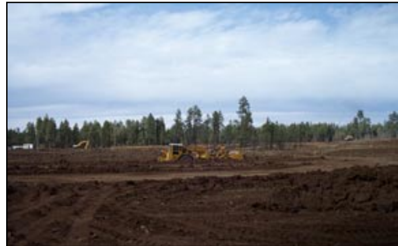
Figure 36: Initial site preparation of the 35 acre Hon Dah wastewater facility, Fort Apache Reservation, Arizona.
