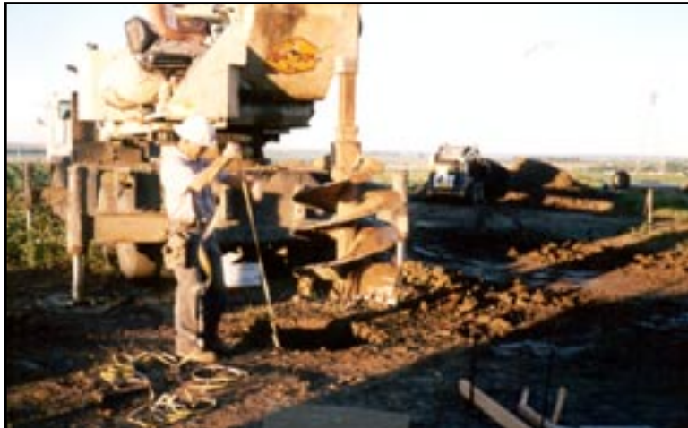
Figure 17: Existing 0.5 acre single-cel lagoon near East Lake, Minnesota.
