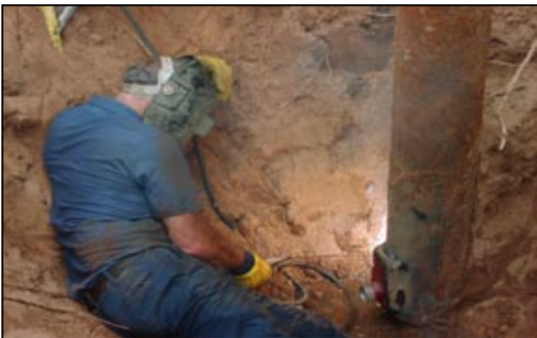
Figure 30: Bernie Nooyan, contractor, welding on a new pitless adapter on the community well for Lac du Flambeau.
