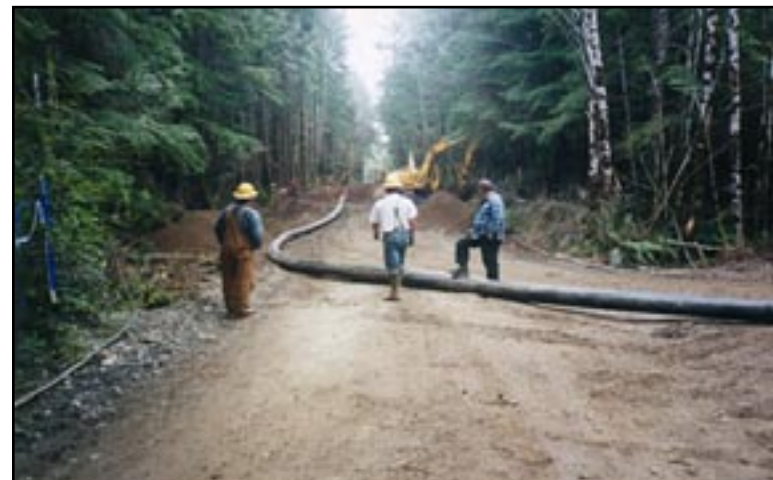
Figure 12: 1Crew installing a 10” HDPE water transmission main on a misty morning on the Quinault Indian Reservation
