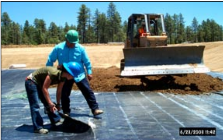
Figure 4: Manuel Quesada and COSTEP Cindi Baxter inspect the liner to ensure the strip of bentonite clay has been adequately applied.
