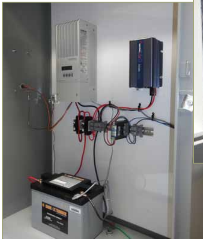
Solar power generation equipment.
