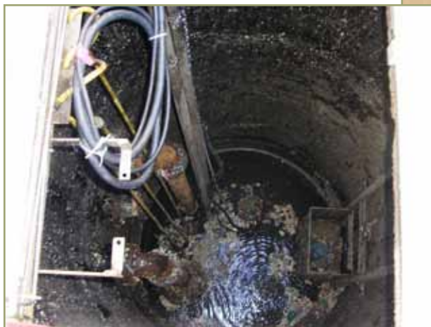
Existing lift station.
