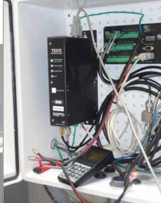
Monitoring equipment inside the pump.
