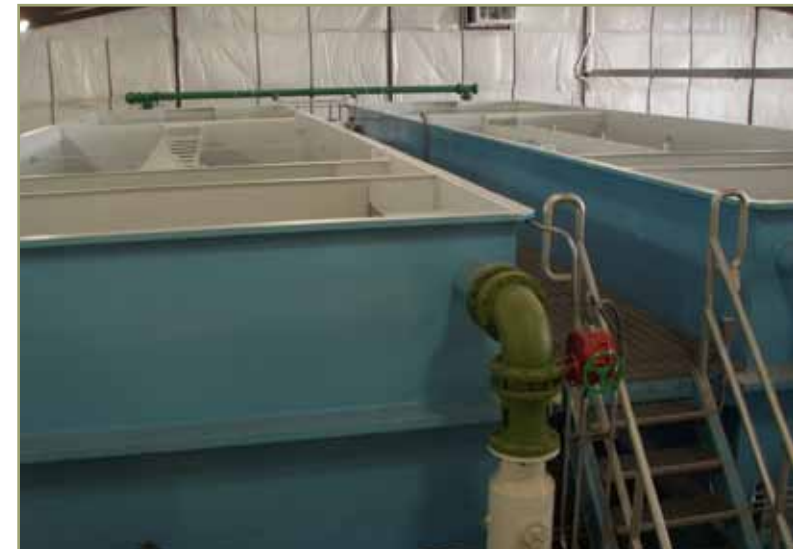
Million gallon per day treatment tanks
