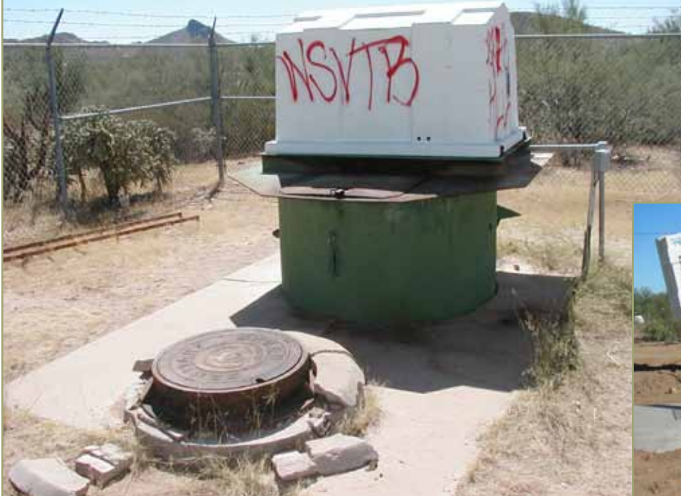
Existing sewage lift station.
