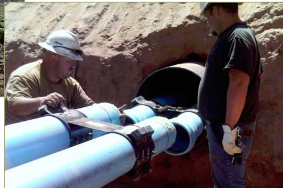
Separate waterline and tank piping.
