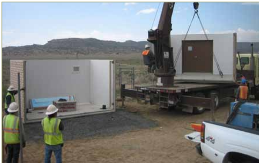
Precast booster pump station, Burnt Corn, Arizona.
