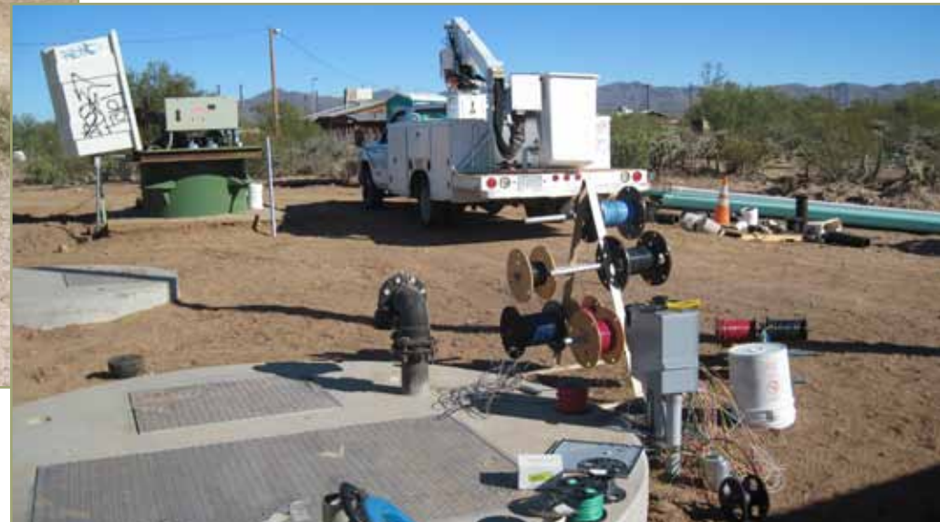
Electrical installation for the sewage lift station.
