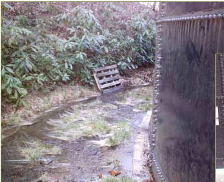
Leaking at the water storage tank.
