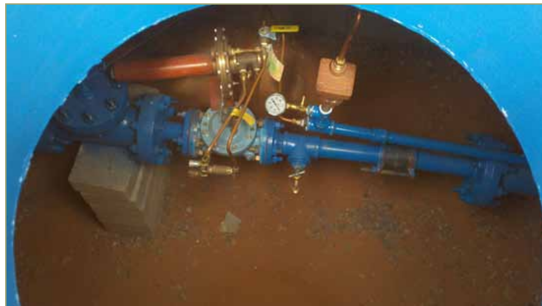
Altitude valve with flow control installed in the Oljato Chapter, Utah.
