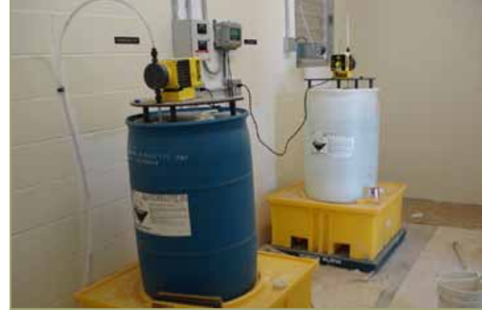
Chemical processing tanks inside the water treatment plant.
