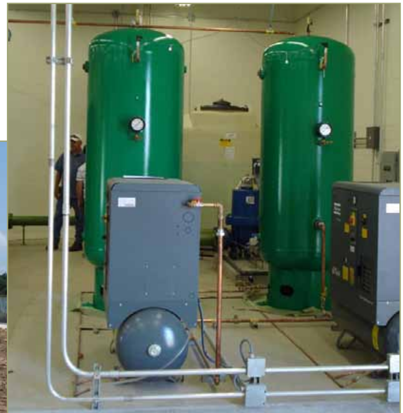
Compressors inside the water treatment building.
