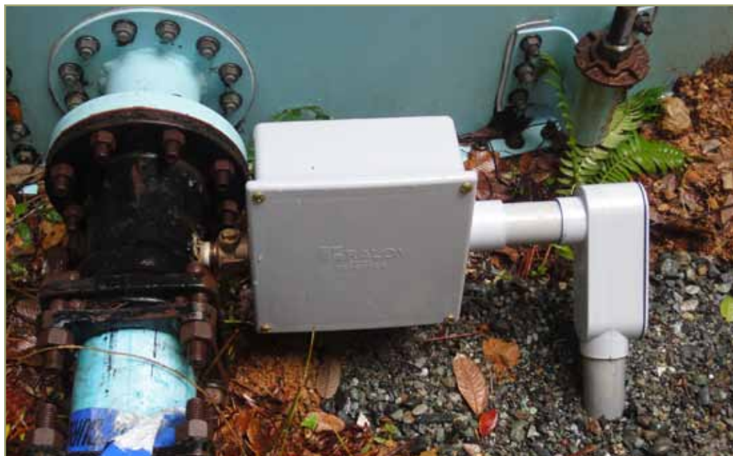
4-20mA water level indicator.
