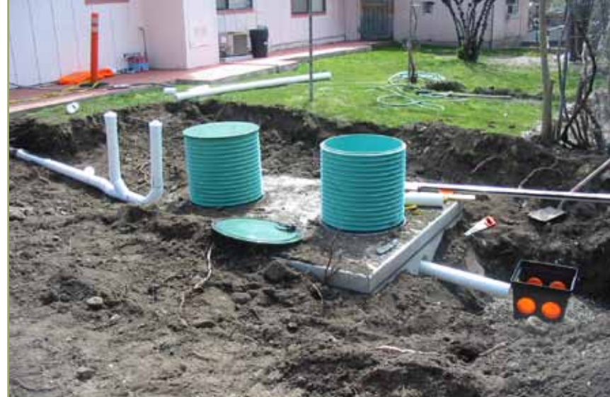
Construction of a septic tank and drainfield system, Santa Ynez Reservation, California.
