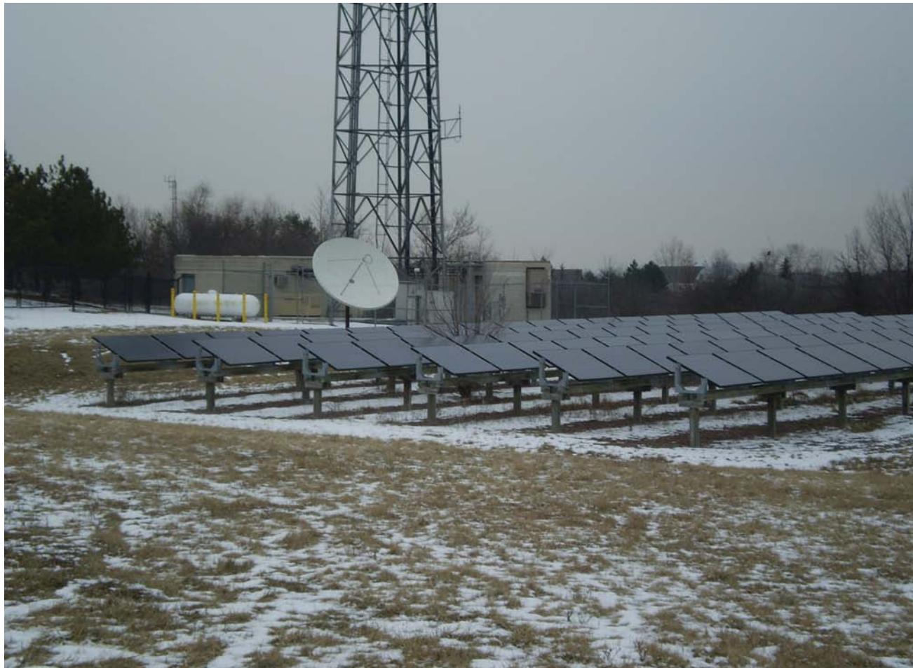
The 100 kW ground-mounted PV system is co-located with an electrical substation in Ann Arbor, Michigan. (Vipin Gupta/PIX179326)
