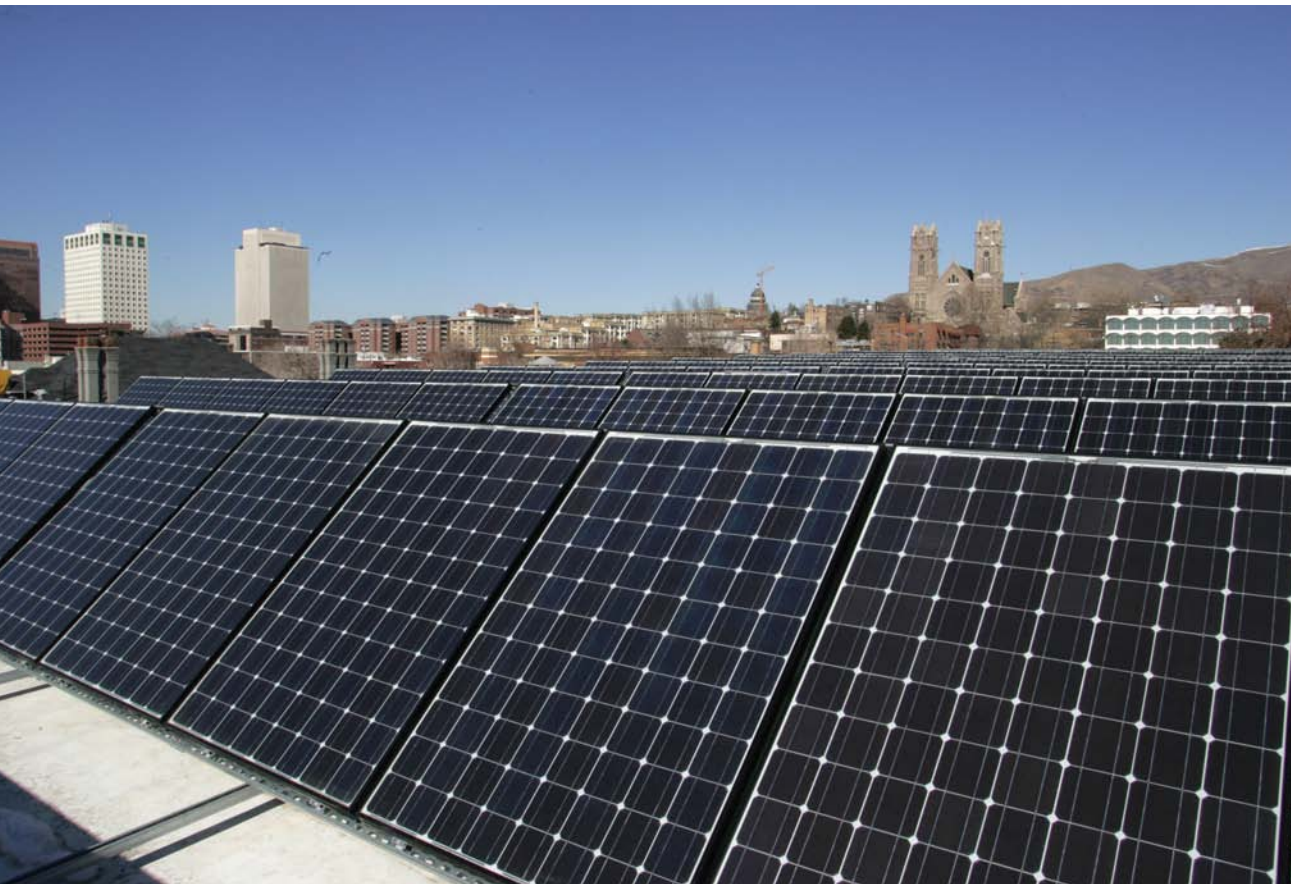
A 25-kW solar PV system provides power to the county-owned Clarke Planetarium in downtown Salt Lake City. (SLC/PIX18364)
